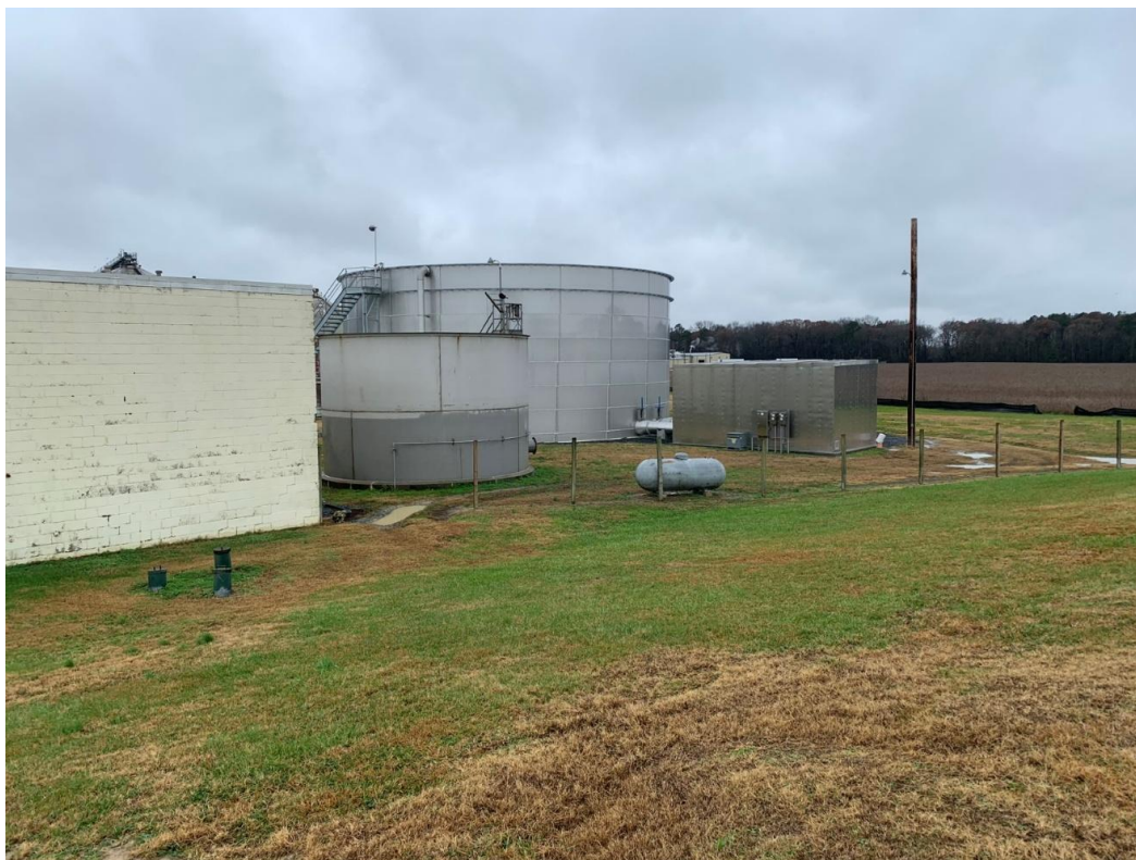
Figure 1. View of the Equalization tank (larger tank) and the DAF sludge tank (smaller)
