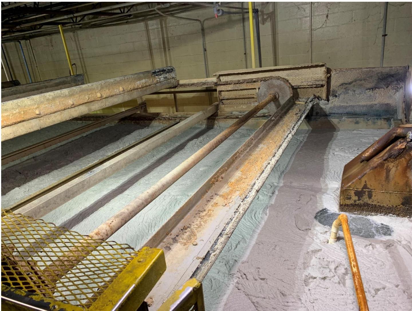
Figure 5. View of the Dissolved Air Flotation Unit from the catwalk
