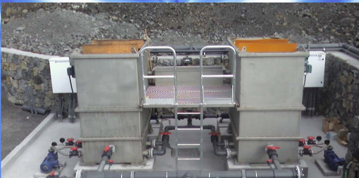
Front View of DAF Units
