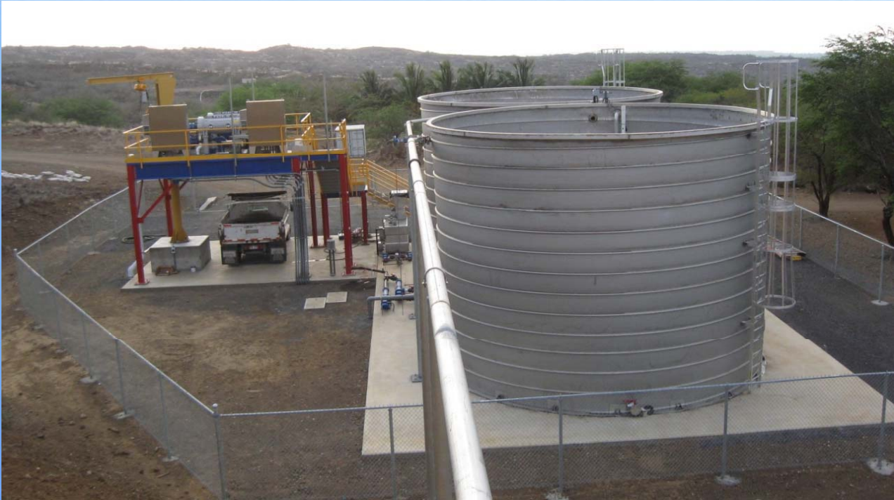
Aerobic Digesters and Centrifuge Dewatering
