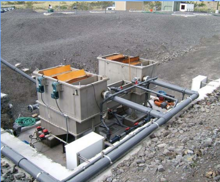
Foreground: DAF Units Background: Below Grade Reactor Tanks
