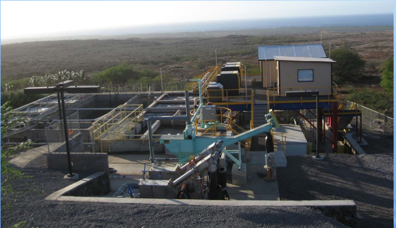
Main Process Area & Upper Mezzanine
