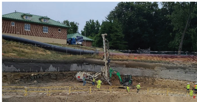
In 2022, a sinkhole near Lake Montebello forced the closure of Whitman Drive. Crews are shown beginning repairs.
