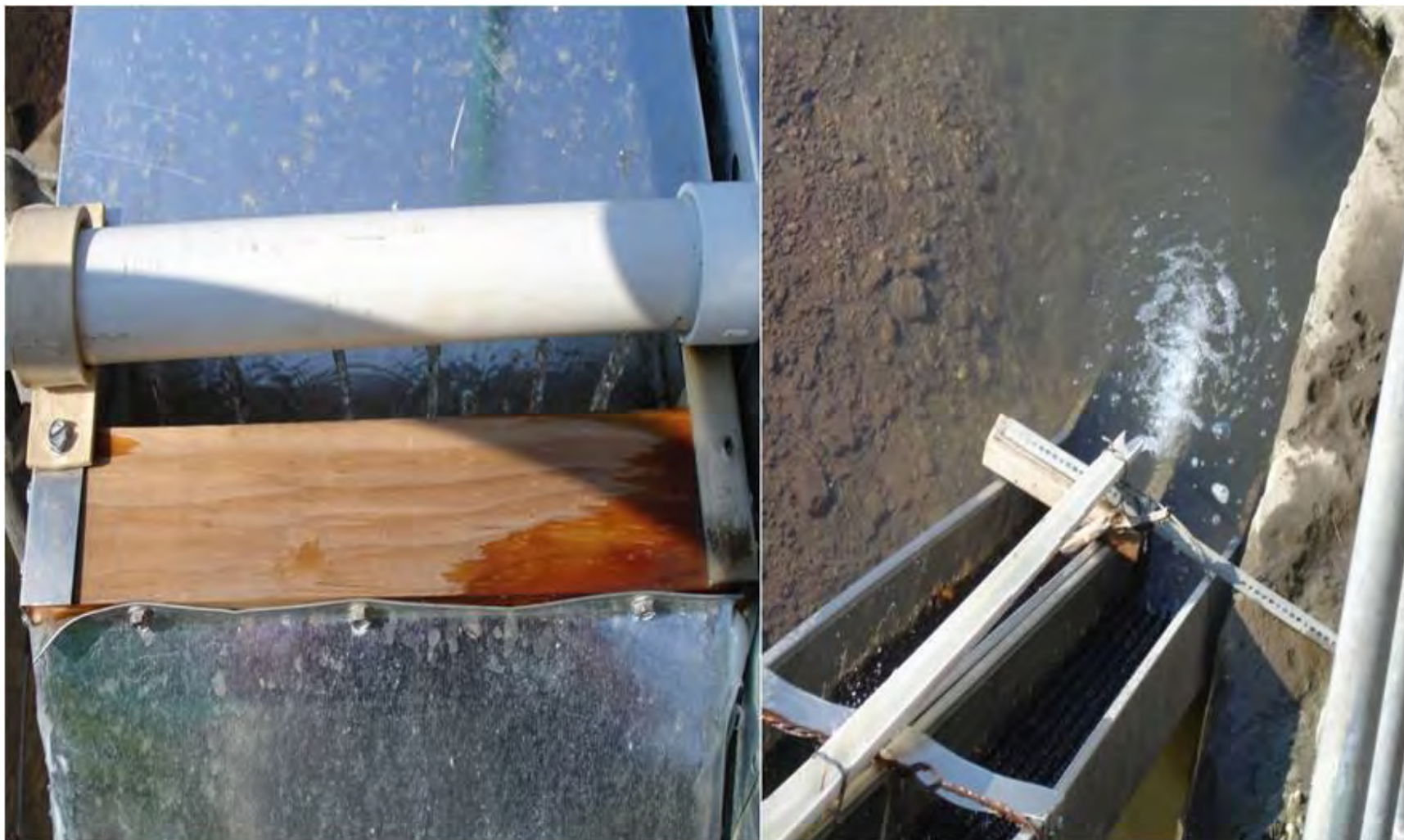
FIGURE 2-9: PHOTO OF SPRAY BAR AND ADDITIONAL FLOW.
