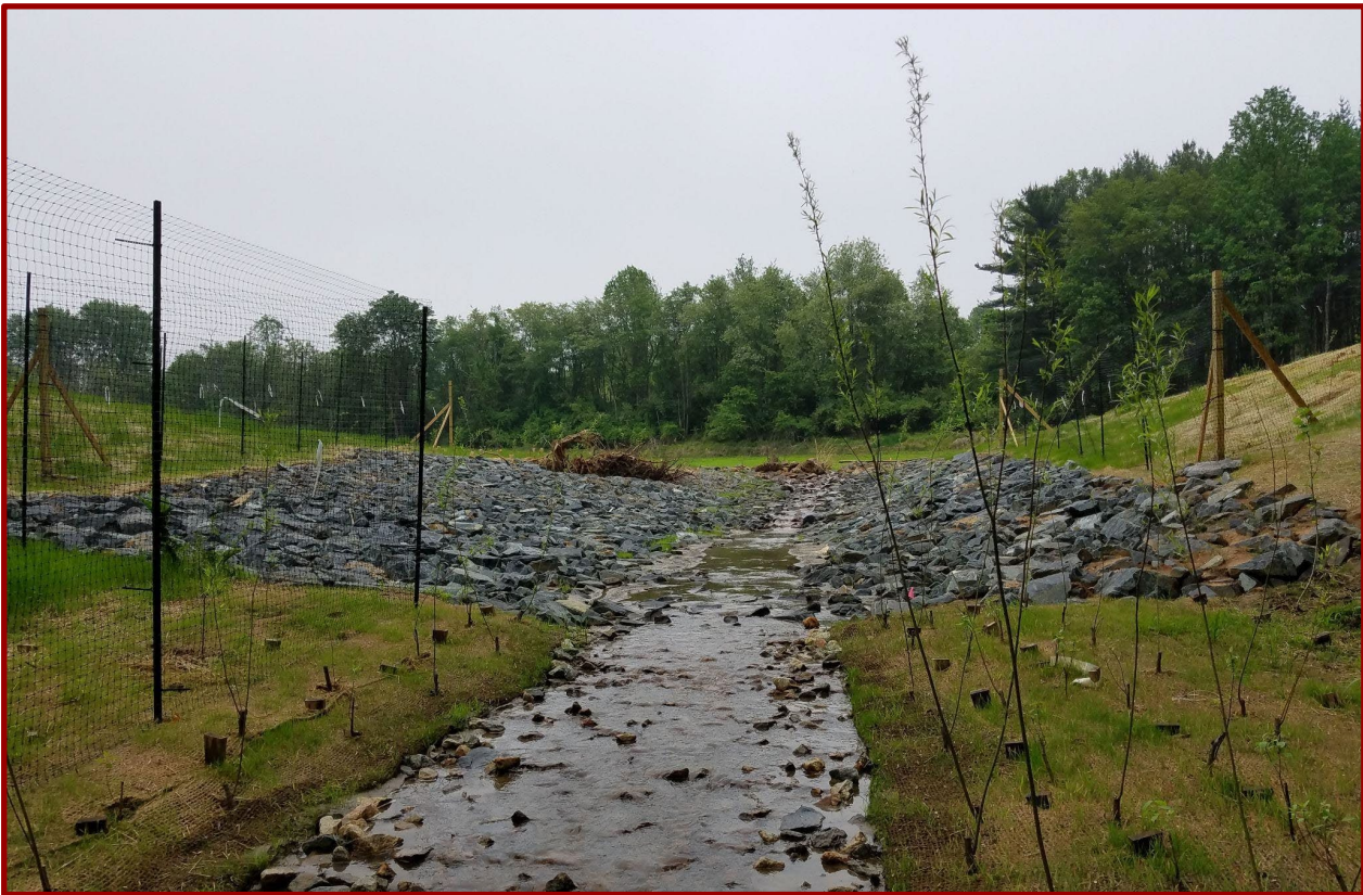
Figure 5.1: MDE photo of stabilized breach channel at former Martin Farm Pond Dam (MD Dam No. 531).
