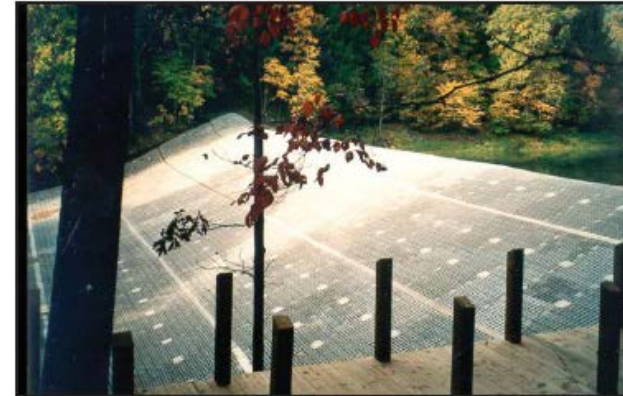
Figure Strahl-6.—Completed view of the cable-tied ACB system at Strahl Lake Dam for overtopping protection. Note all joints have been grouted (Courtesy of Contech Engineering Solutions, all rights reserved).
