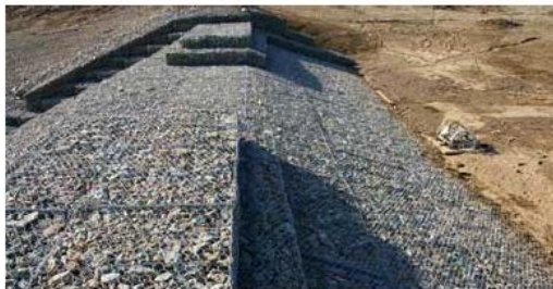
Figure 5-4.—Example of gabion spillway crest structure. (Courtesy of Concorib, all rights reserved)
