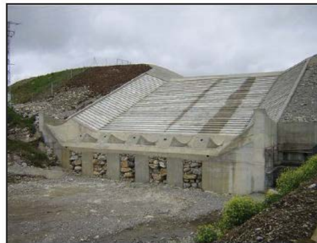
Figure Barriga-14.—Completed spillway prior to operation (courtesy of Morán and Toledo, 2006, all rights reserved).
