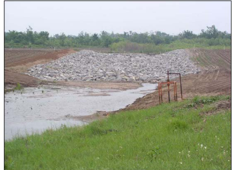
Figure 8-2.—Rock chute spillway on Little Washita Site 13 in Grady County, Oklahoma. This chute was installed in 2010 to convey flows over the remnants of the decommissioned dam (USDA-NRCS, Courtesy of Chris Stoner).
