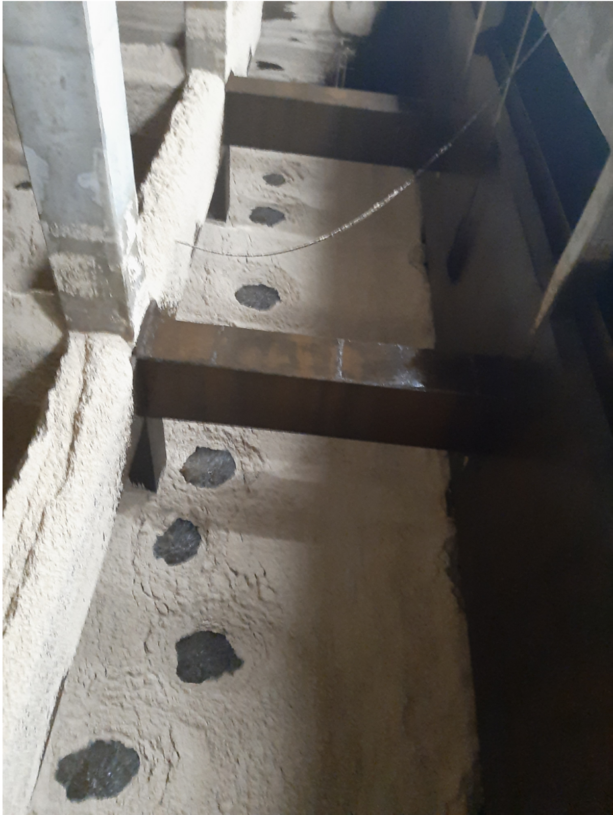
11/2/22 Picture of backwash mud well showing media accumulation. Effluent from the mud wells goes to Secondary Clarifier #3.
