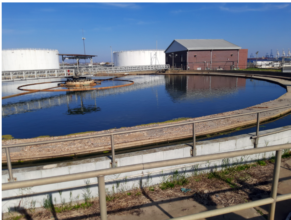
Secondary clarifier #1 note debris on the launder covers.
