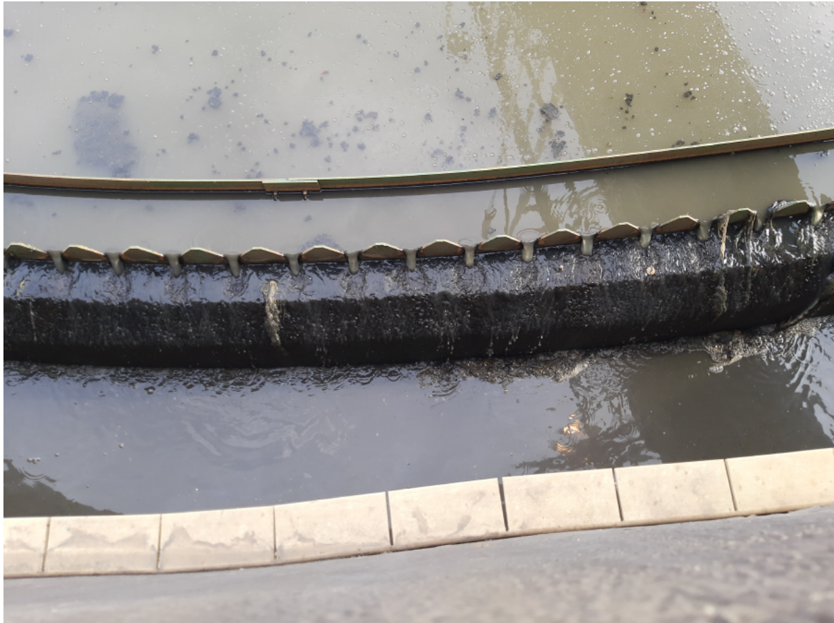
11/2/22 GST #2 rags on the weirs and media floating on the surface.
