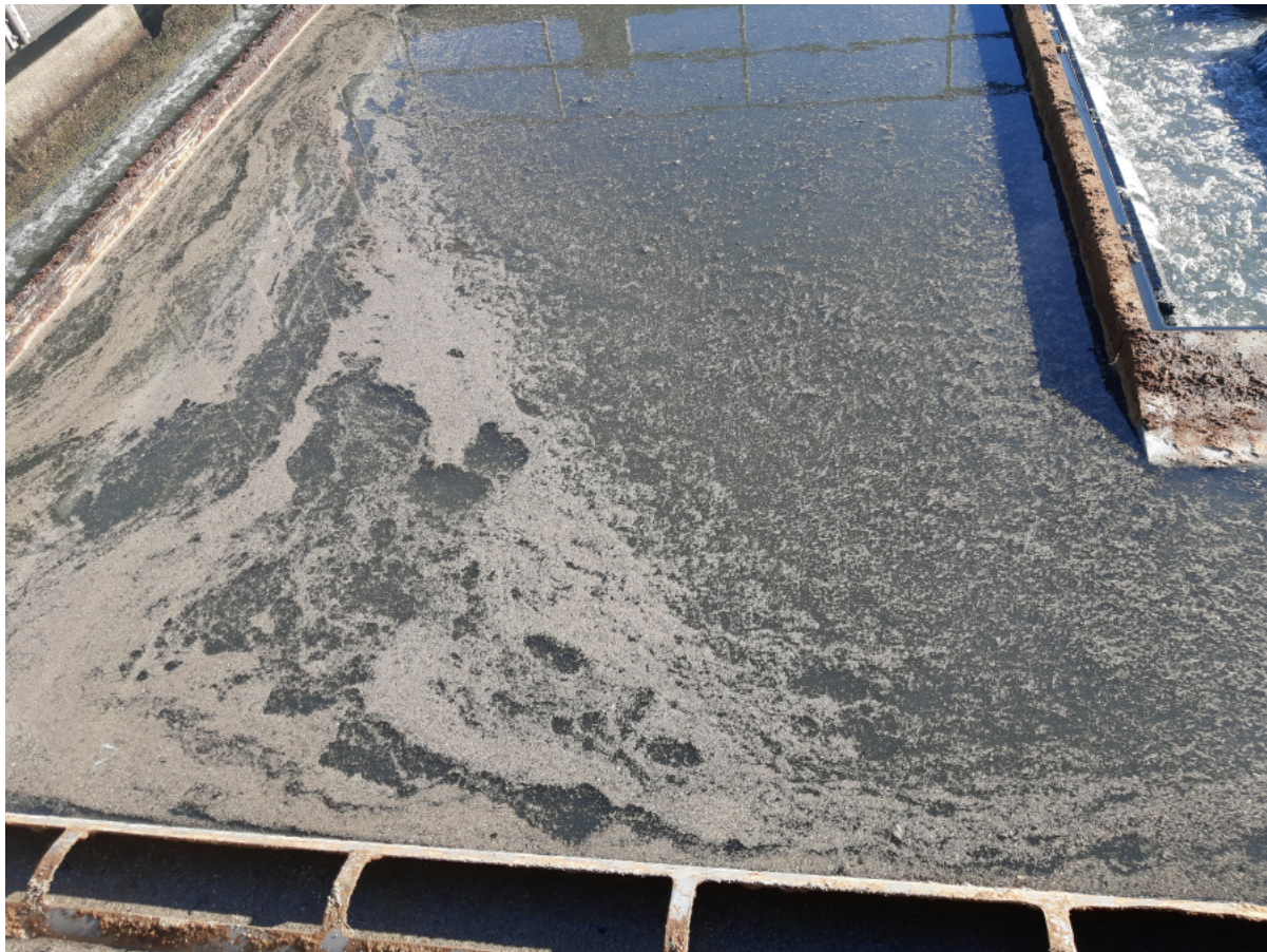
11/2/22 PST #1 Note the floating media and scum.
