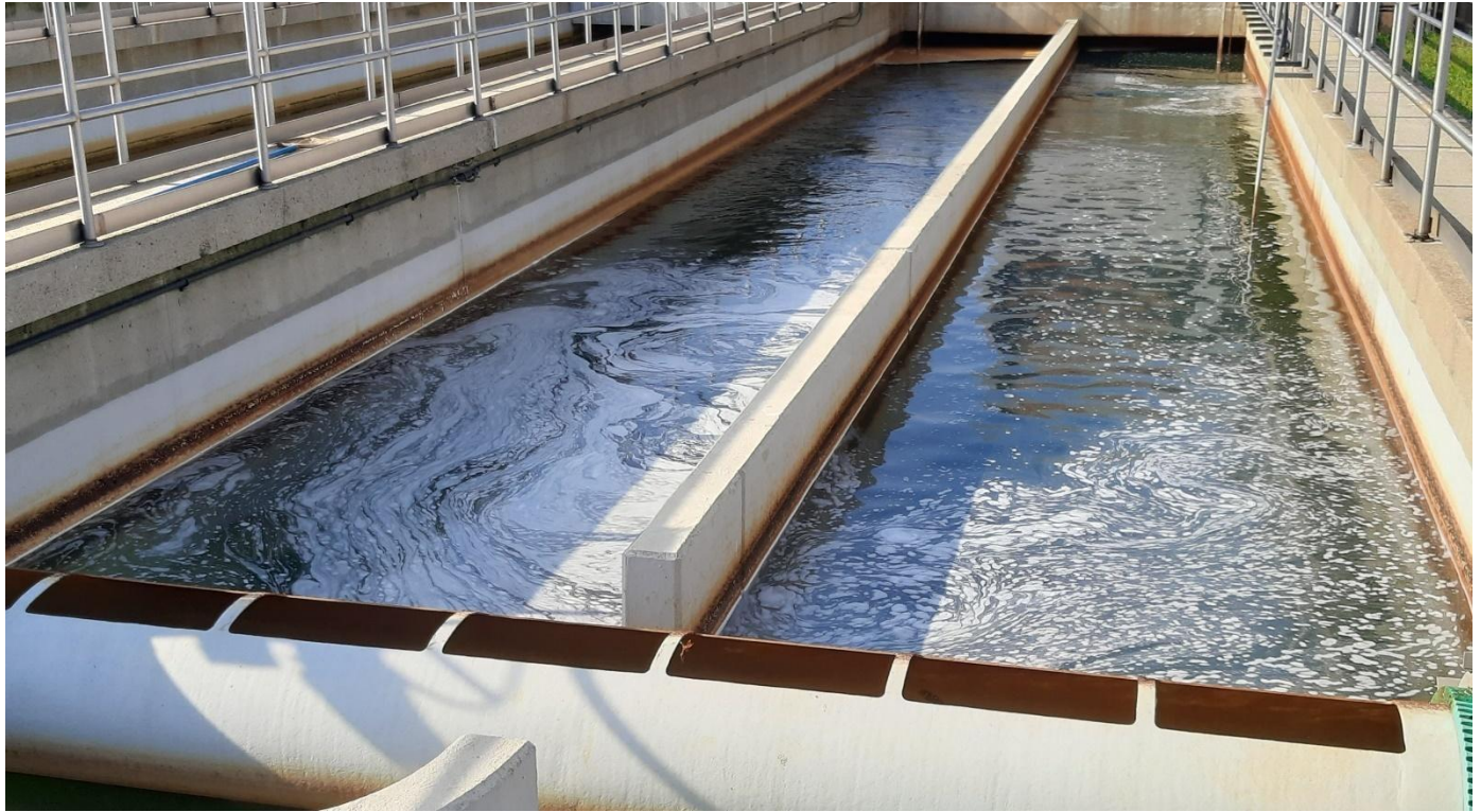
11/2/22 Chlorine contact basin. The water level is at an appropriate height to rotate the scum log in order to collect the floating FOG/scum.
