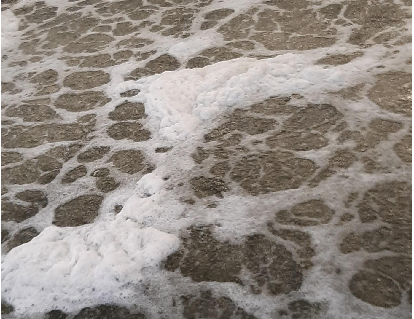
11/2/22 BAF cell #5 heavy foaming due to BOD level.
