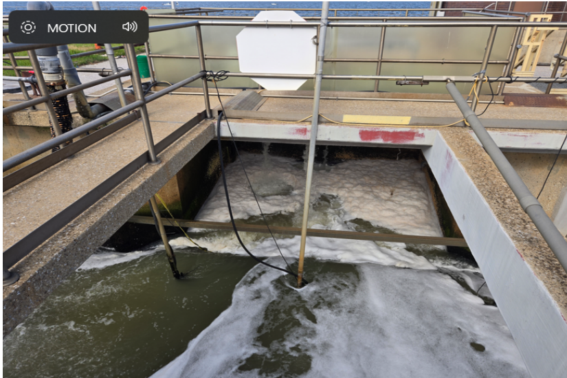
Image 03: Final effluent discharge with persistent foam
