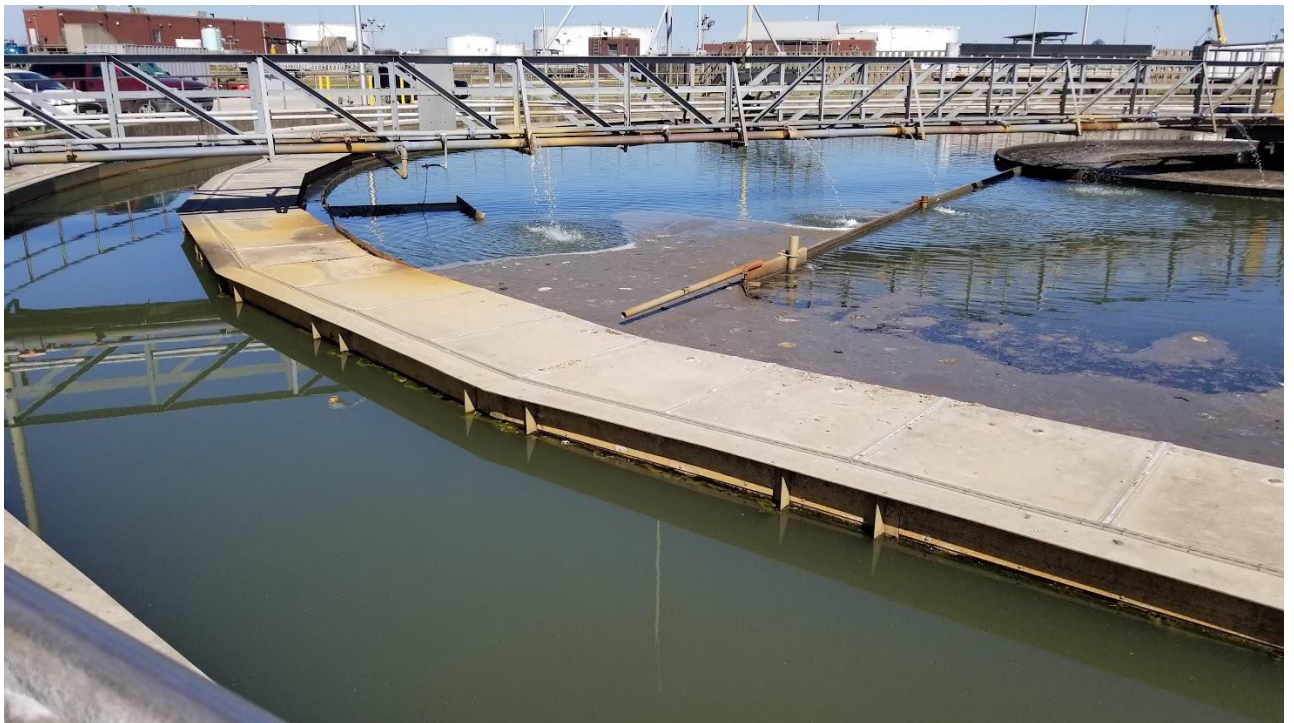
Figure 2f: Scraper arm in Clarifier # 5A is missing.
