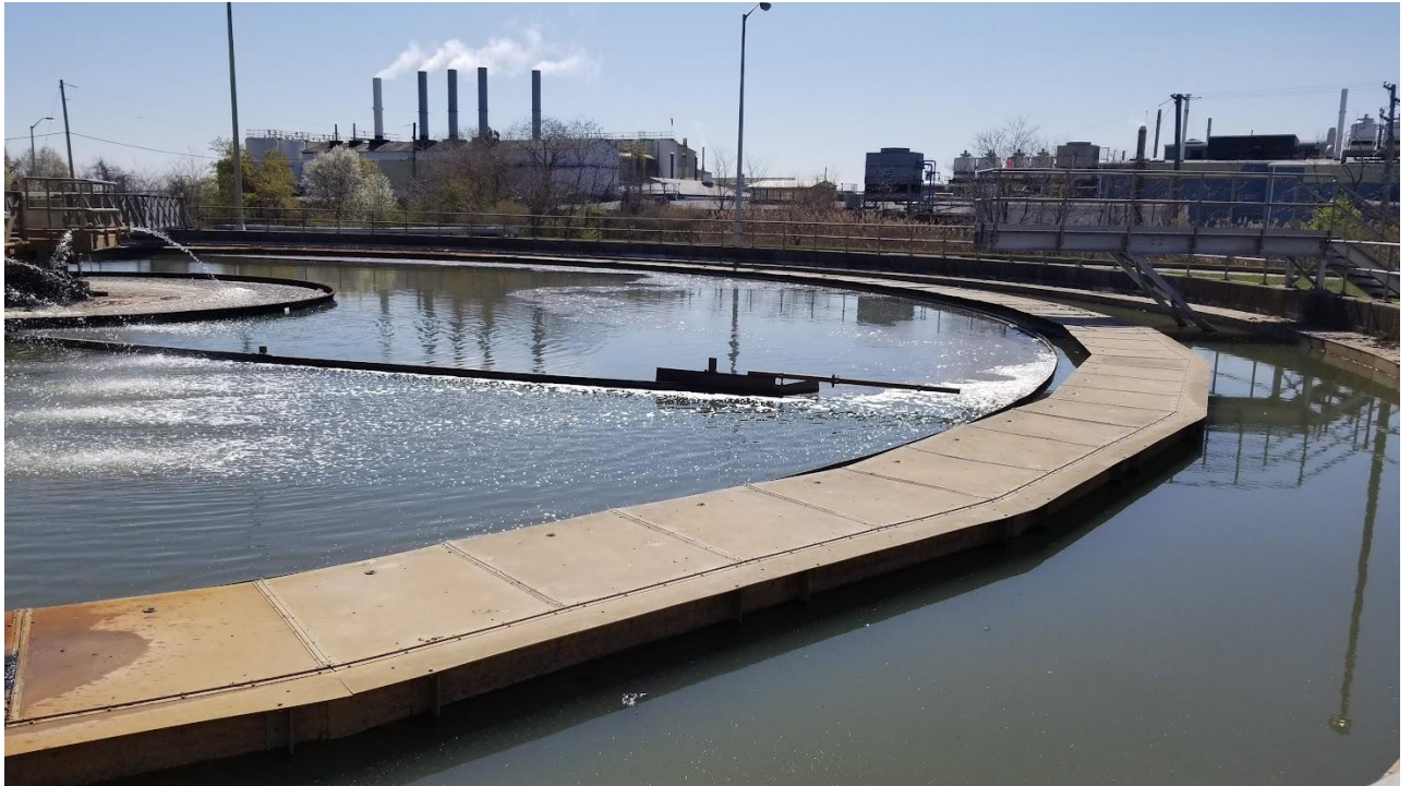
Figure 2e: Scraper arm in Clarifier # 5B is missing.
