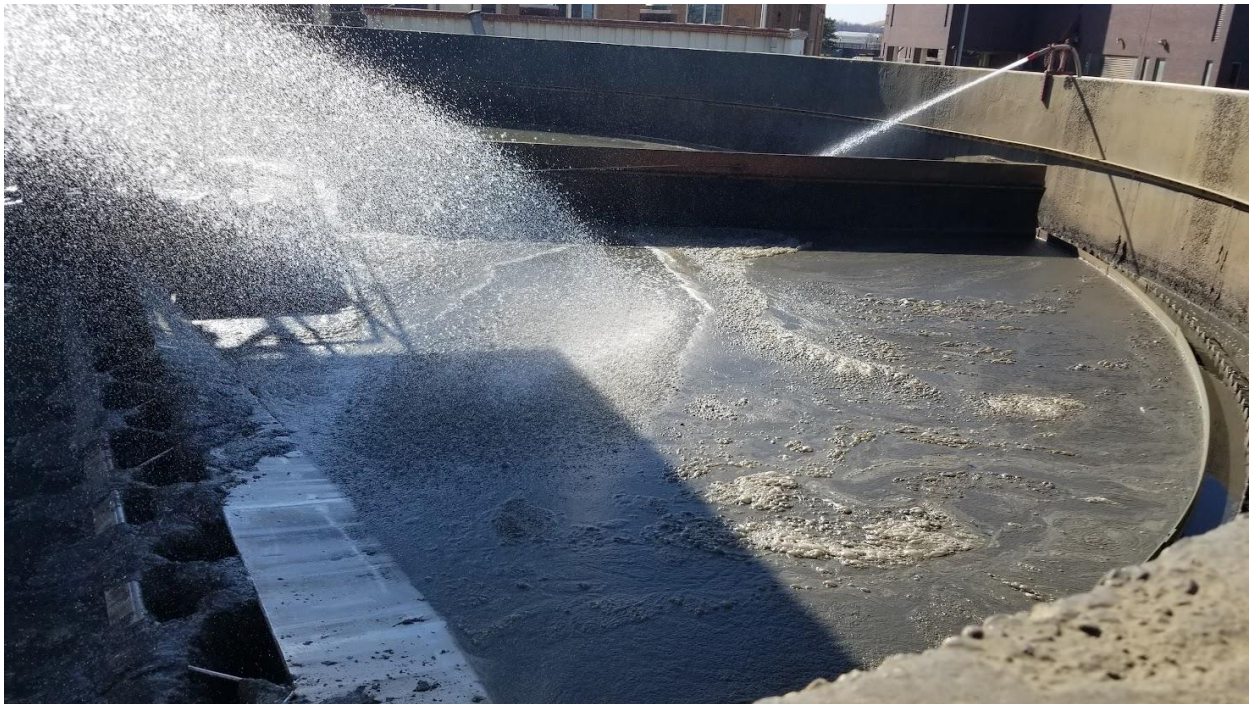
Figure 1d: Sludge on the surface of GST #2.
