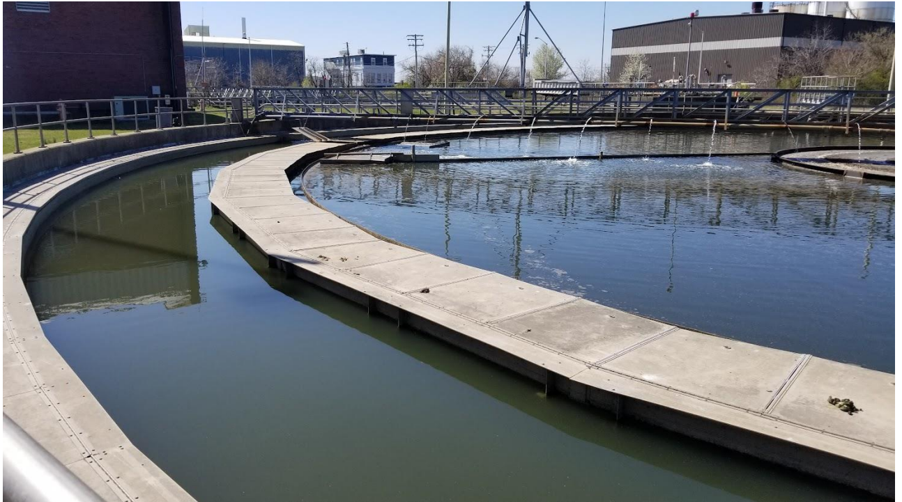
Figure 2c: Rubber part of the scraper arm in Clarifier #6A is missing.
