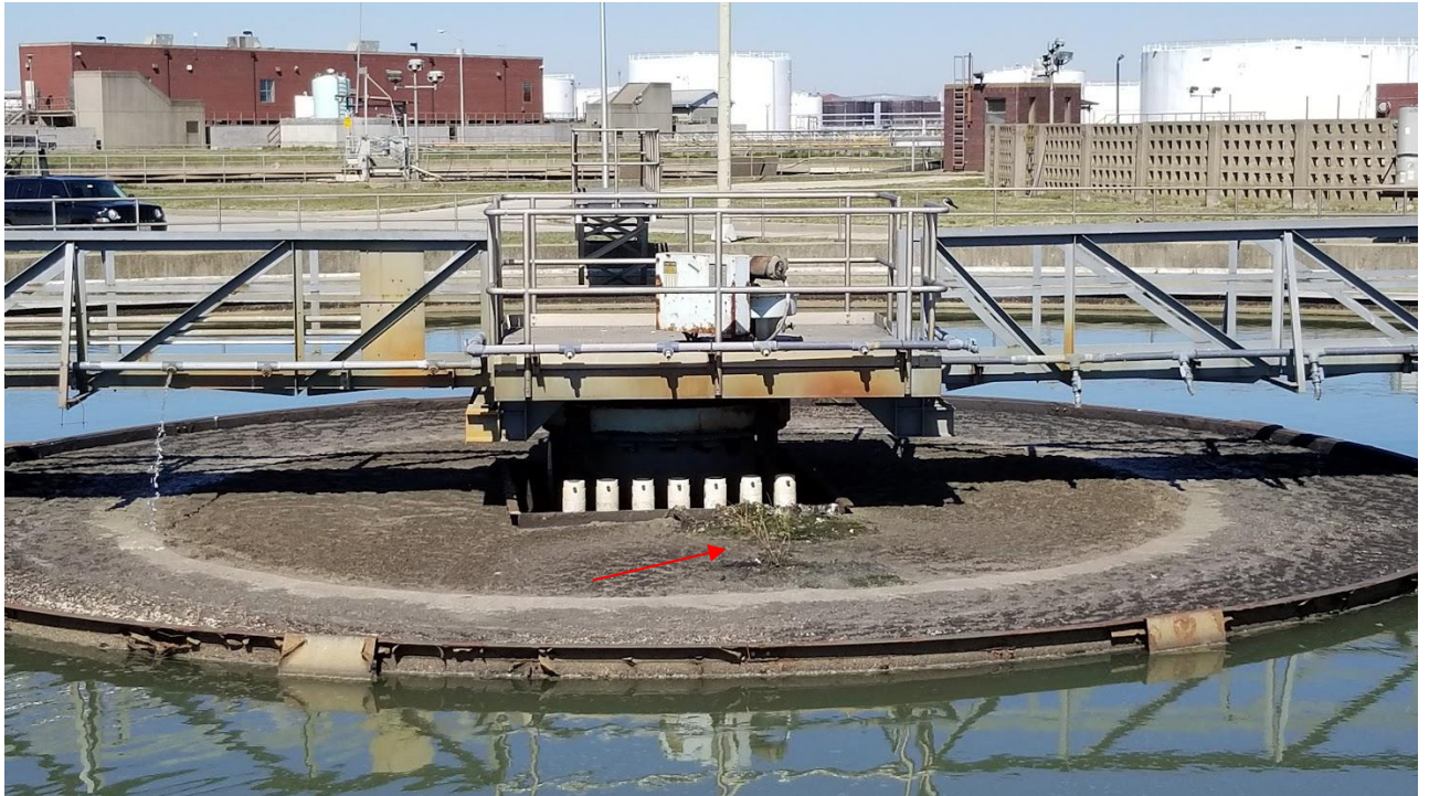
Figure 2g: Woody vegetation in the center of Clarifier # 5A (pointed out with a red arrow).
