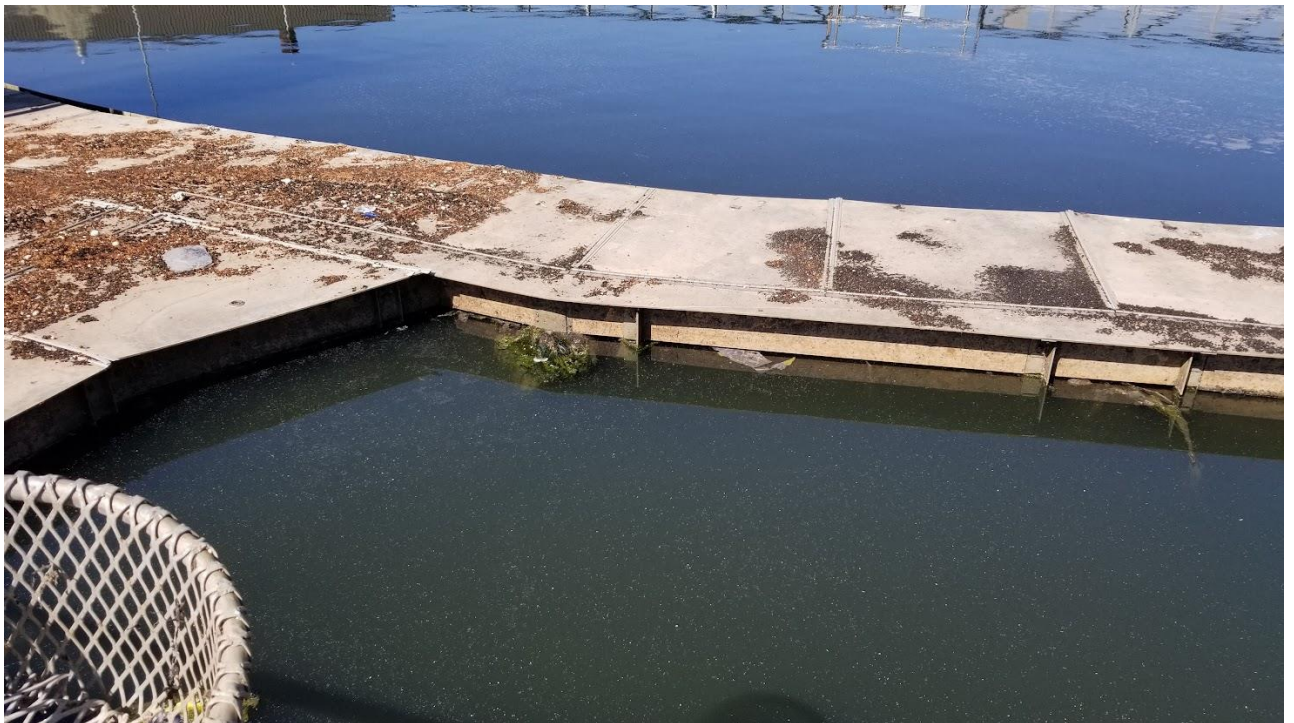
Figure 2d: Solids outside of launder cover within Clarifier # 6B.
