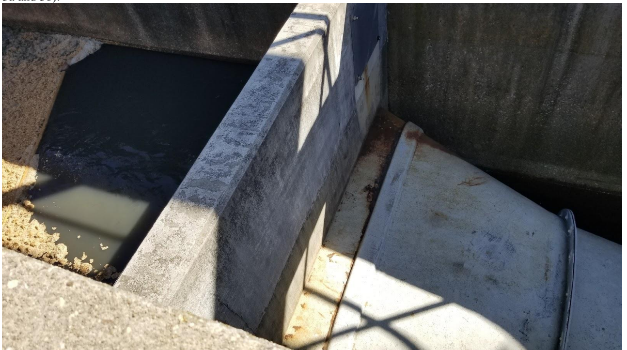
Figure 3a: FOG backflowing into the outflow side of PST and inflow side of the pure oxygen reactors.
