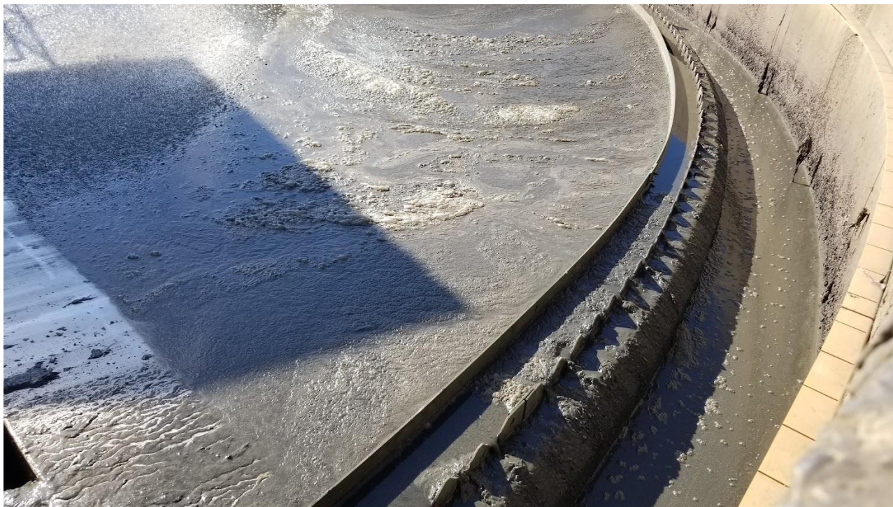
Figure 1e: Sludge next to the V- notch weir at GST #2.
