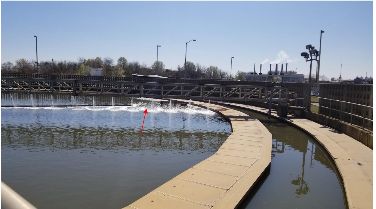
Figure 2a: Scraper arm of Clarifier #4 is missing. The red arrow shows the gap between scum skimmer and the weir.
