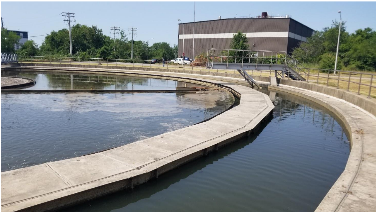
Figure 5f: The rubber part of the skimmer arm in Clarifier # 6B is not leveled and is partially submerged in water.
