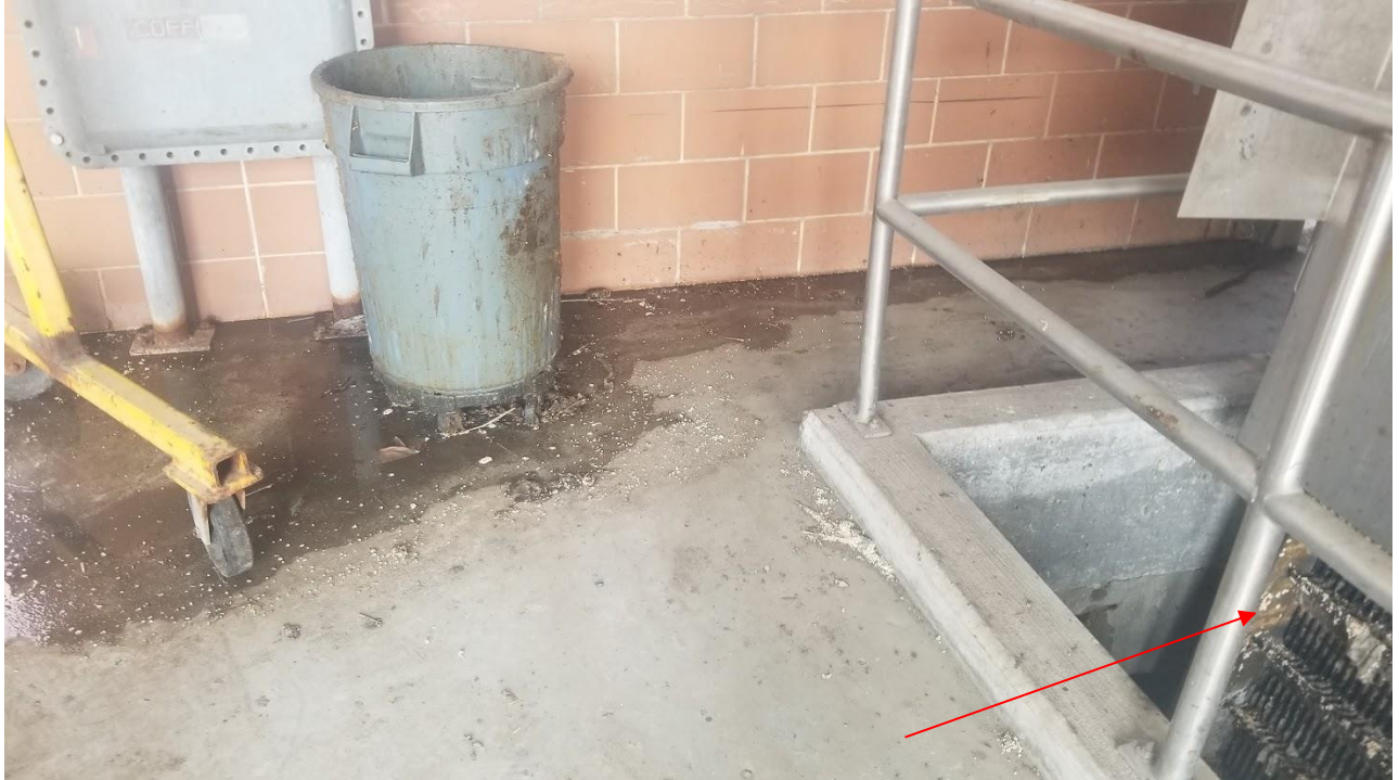
Figure 1b: BAF media on the ground by bar screen #1 inside the west side of the IPI building. There are some BAF media on bar screen #1 (pointed to with a red arrow).
