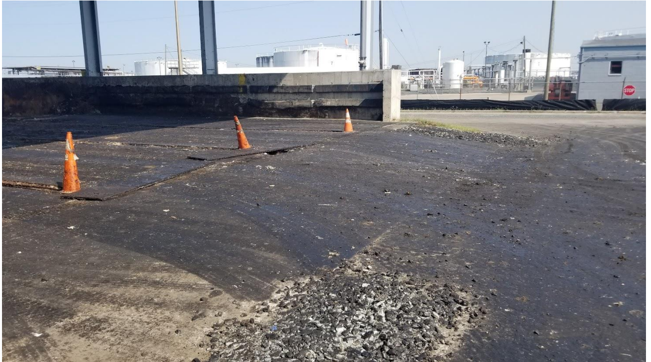
Figure 2a: Grease track at the transfer station facing northwest.
