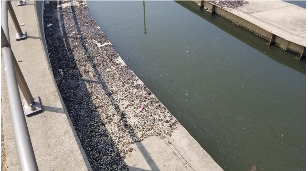
Figure 5g: Media on launder cover of Clarifier #6B.
