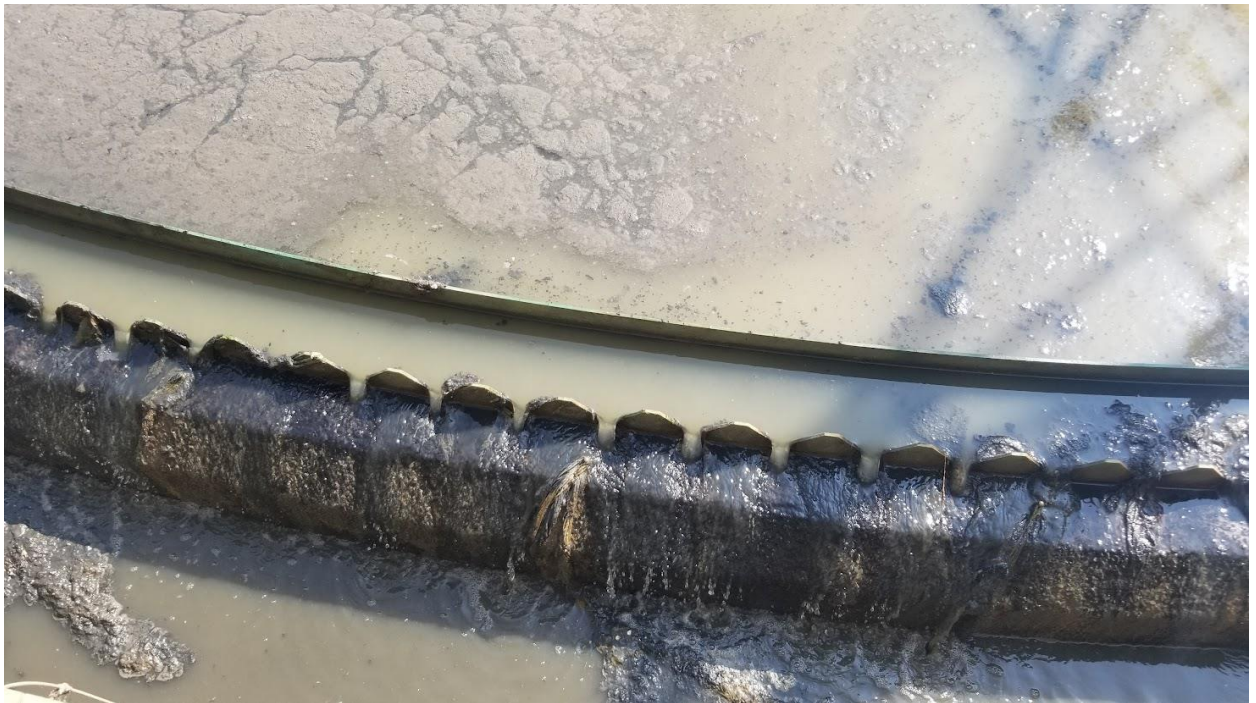
Figure 3b: Sludge outside of the weir in GST #1.
