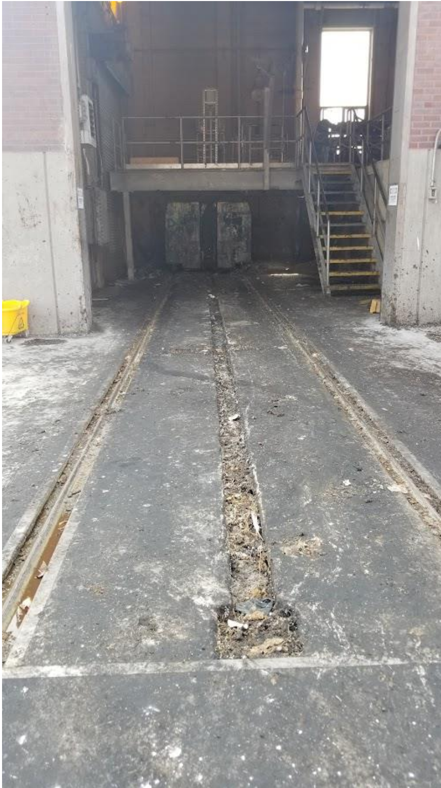
Figure 2d: View of the northwest side of the combined influent building (location of potential grease and grit from fine screens #1- 4 would be dropped into dumpsters at the output side of the conveyor). There are some media imbedded along the depressed area in the middle of the picture.
