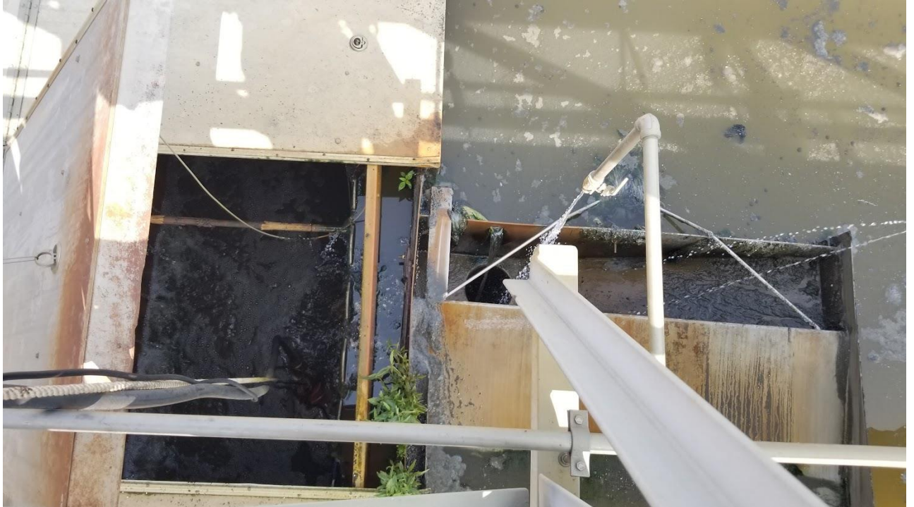
Figure 5a: Plants in Clarifier #1, by the V- notch weir
