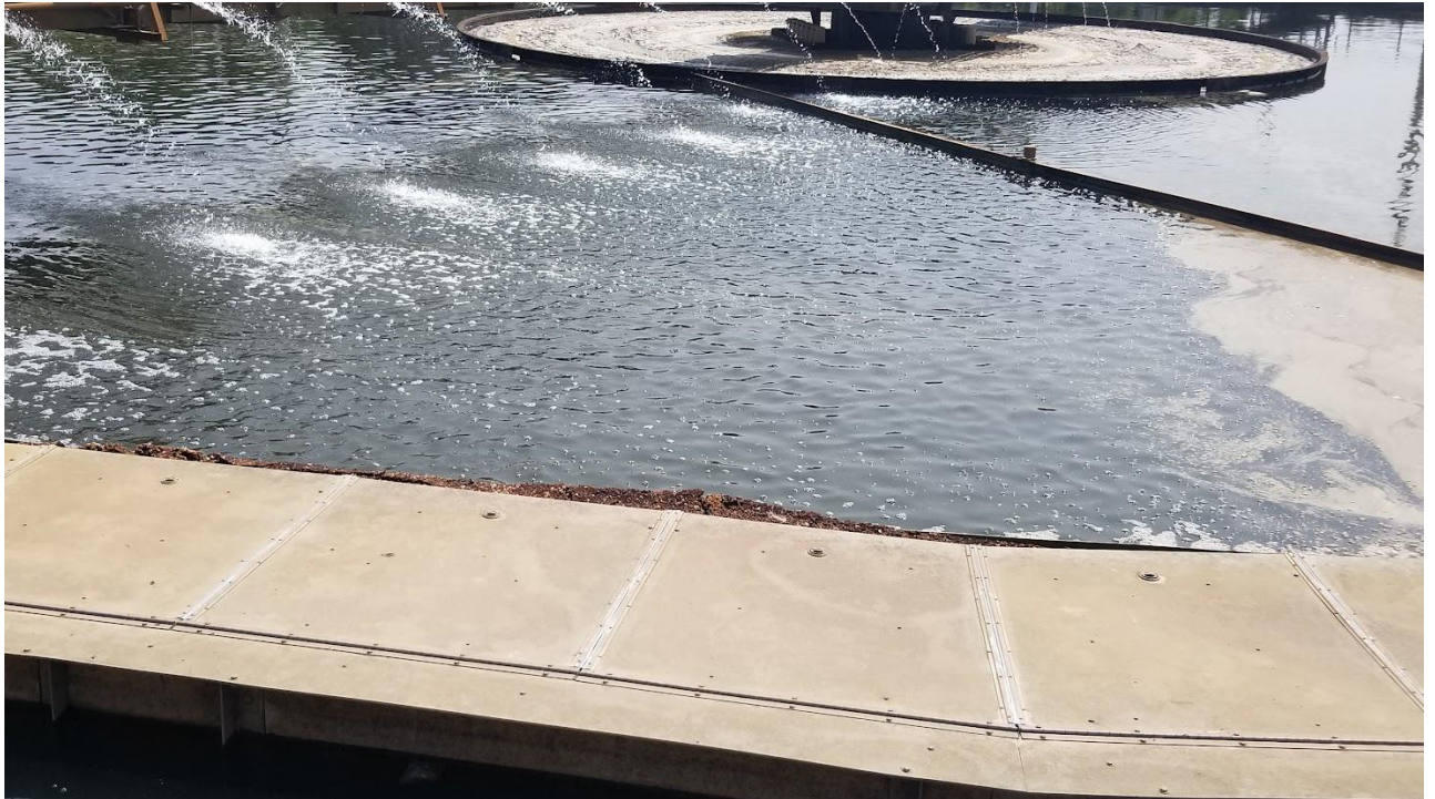
Figure 5k: Close up view of the debris shown in Figure 5j, with debris above the height of the baffle in Clarifier #5B.
