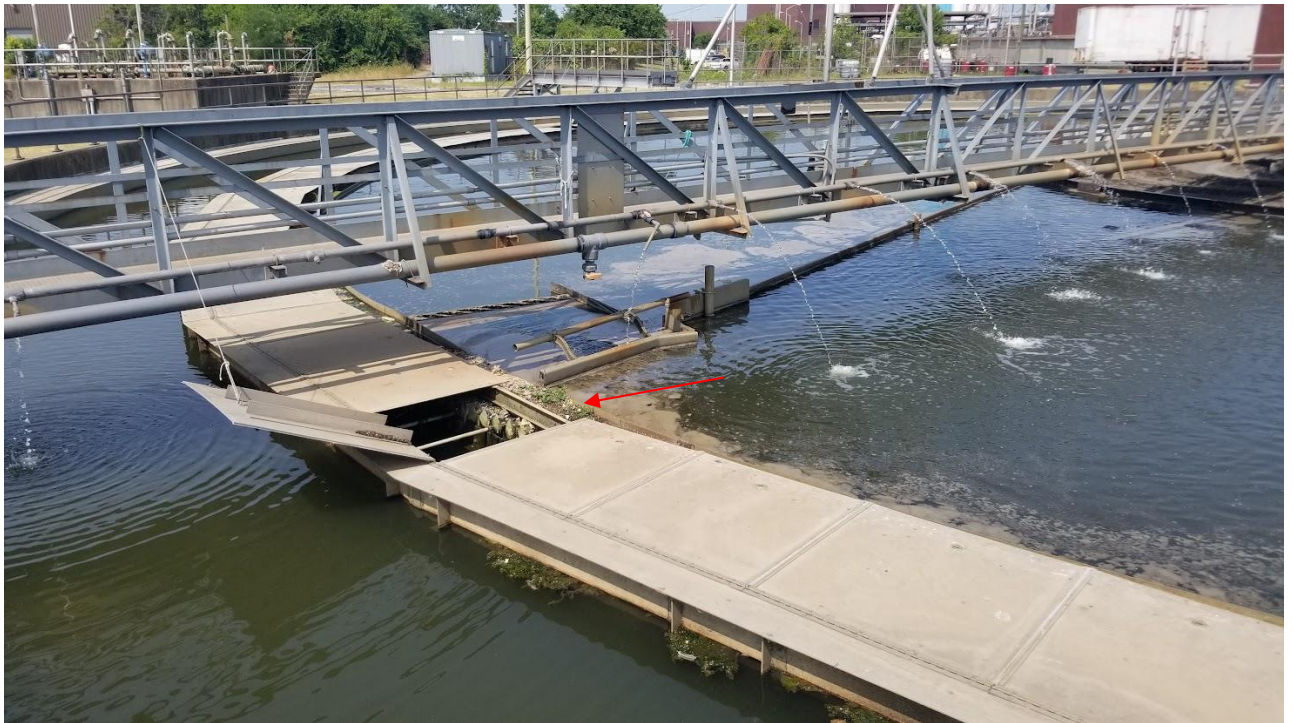
Figure 5d: Plant and debris by the launder cover in Clarifier # 6a (pointed to with a red arrow).
