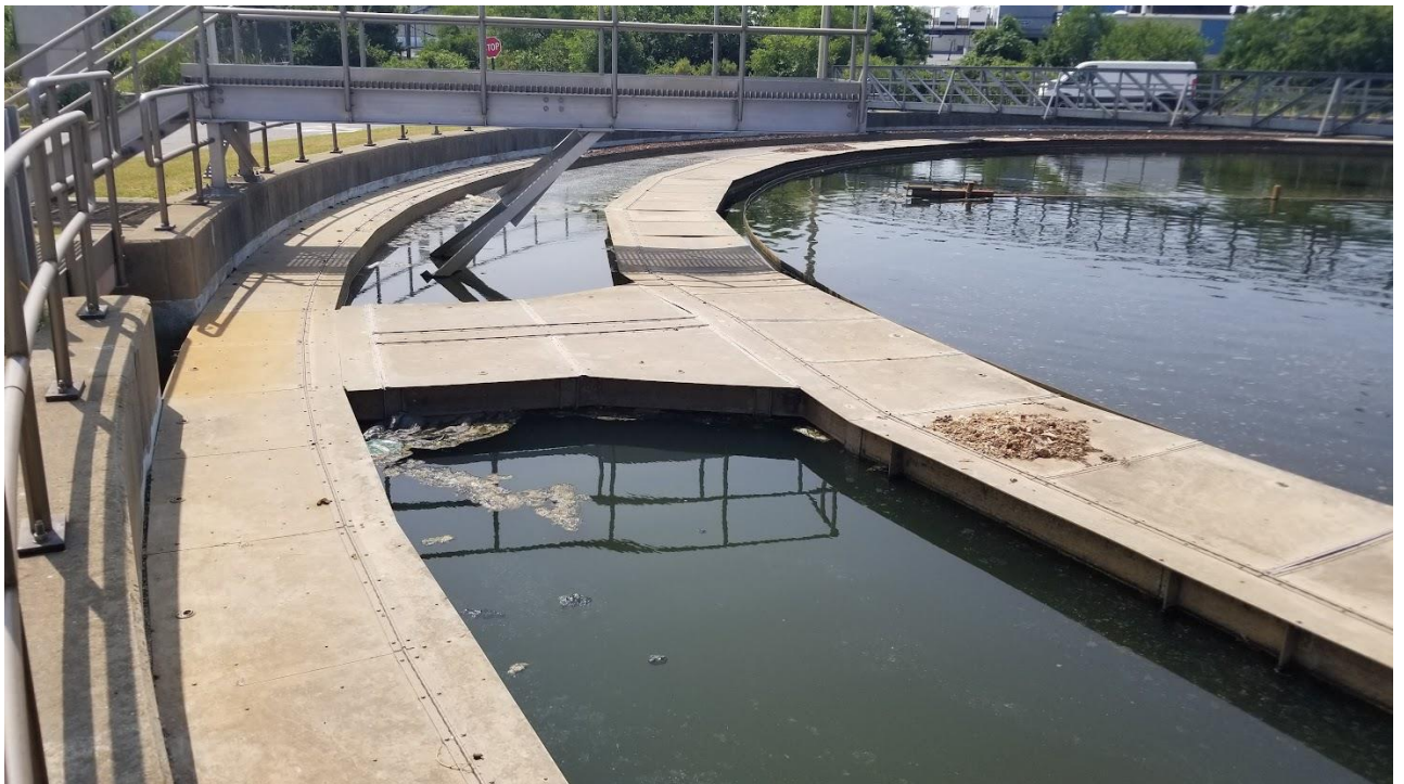
Figure 5l: Trash in Clarifier # 5B and a section of the scraper arm is missing.
