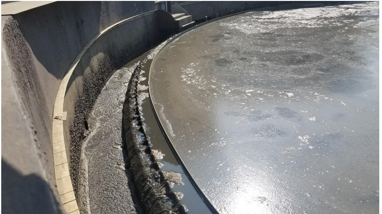
Figure 3c: Sludge outside of the weir in GST # 2.
