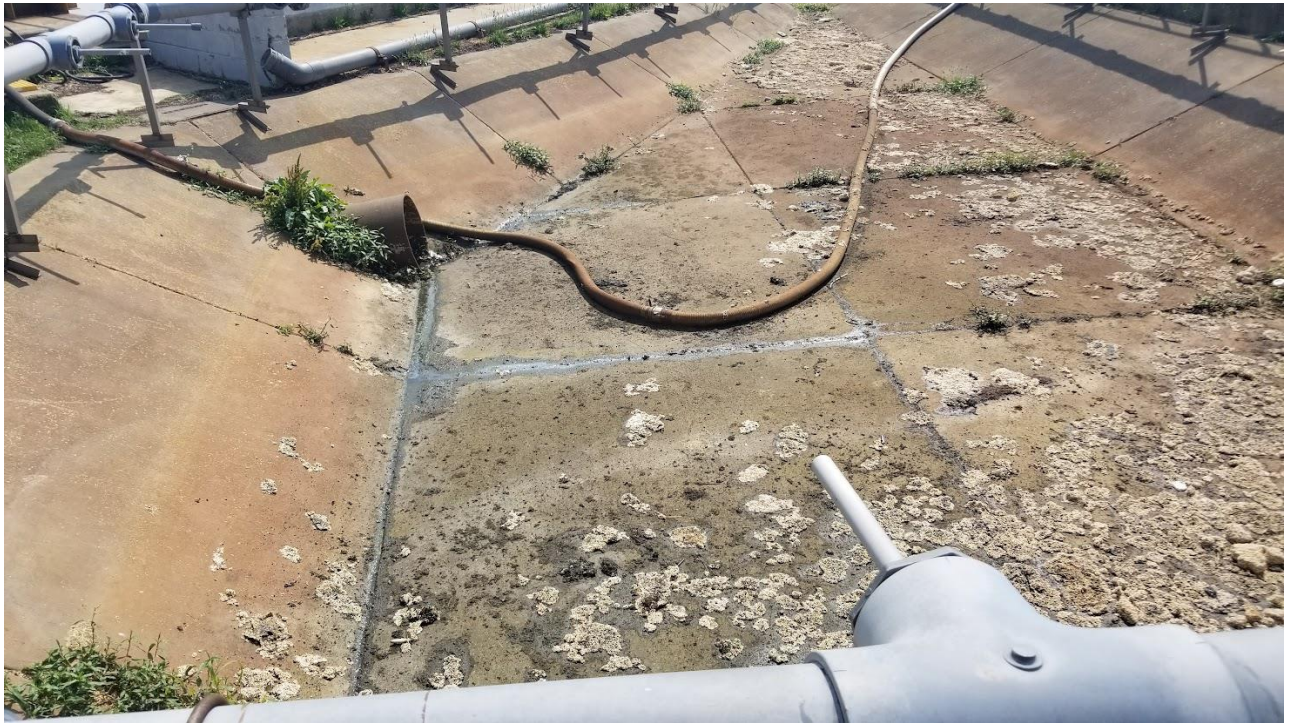
Figure 4a: BAF media in an outflow pit by the southwest side of Clarifier #1 facing northeast.
