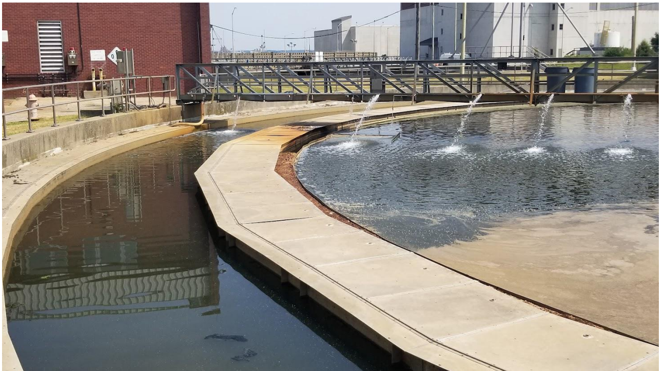
Figure 5j: Debris between the launder cover and baffle of Clarifier #5B.
