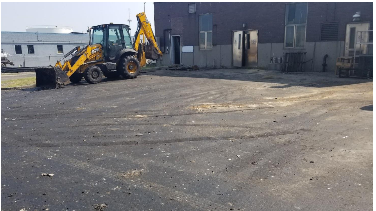
Figure 2b: Grease track and grit on the ground by the transfer station. This location is immediately east of the area shown in Figure 2a, facing northeast.
