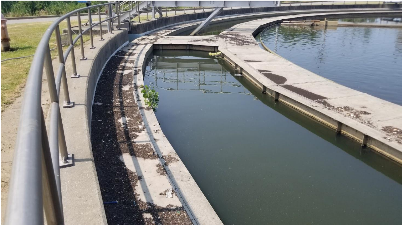
Figure 5i: Plant growing by the launder covers in Clarifier # 6B.
