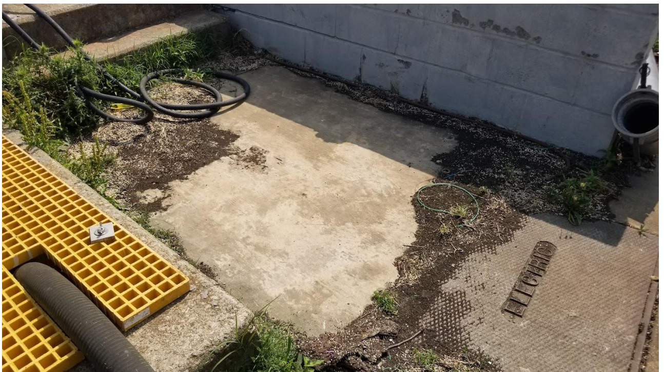
Figure 4b: BAF media on the ground by the stairs leading to the south side of Clarifier #1.
