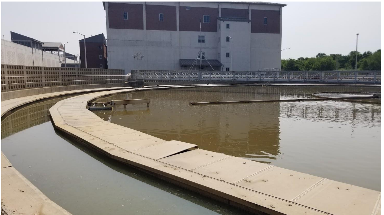
Figure 5b: A section of the skimmer arm in Clarifier #4 is missing.
