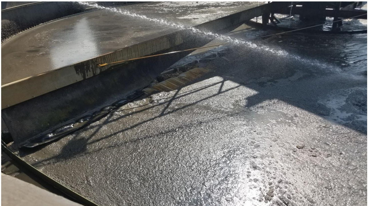
Figure 3d: Excessive amount of sludge in GST # 2.
