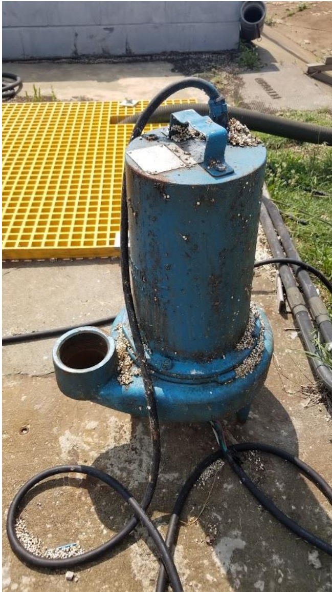
Figure 4c: BAF media on the ground and a pump by the south side of Clarifier #1.
