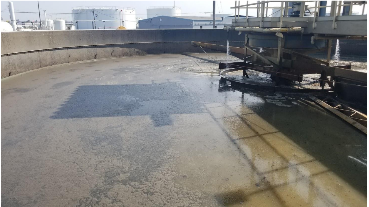
Figure 3a: Excessive amount of sludge in GST #1. A skimmer arm in GST #1 is above the water surface.
