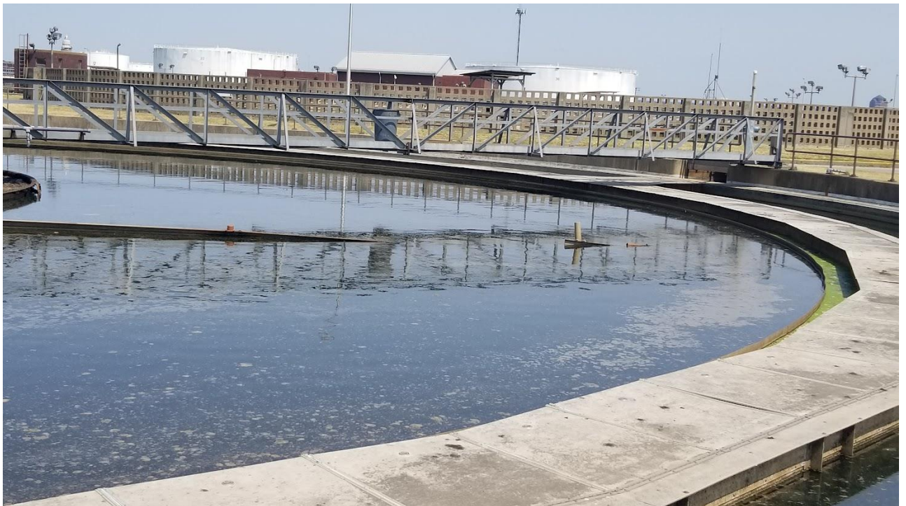
Figure 5n: A skimmer arm partially under water in Clarifier 5A.
