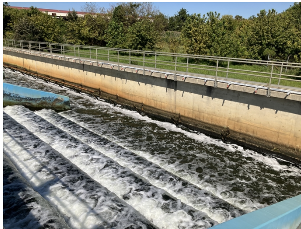
Image 03: Step Aeration system, final effluent.
