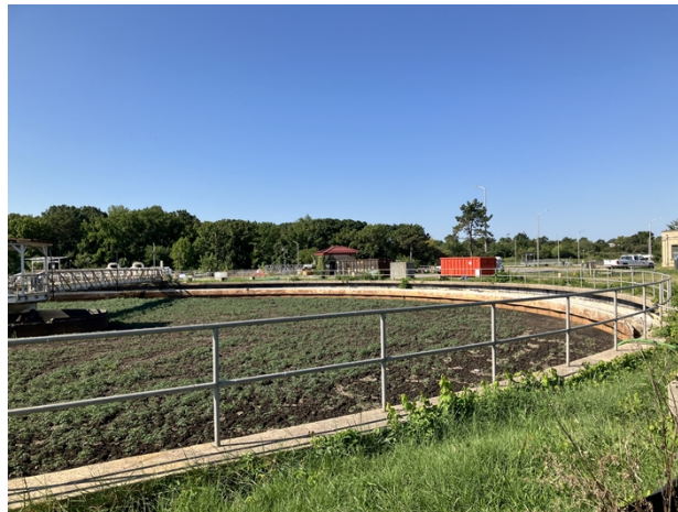
Image 02: PST # 1, drain line clogged.
