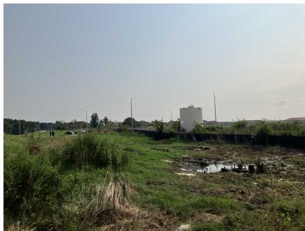
Image 06: Area of the sludge cleanout, uprights near standing water.
