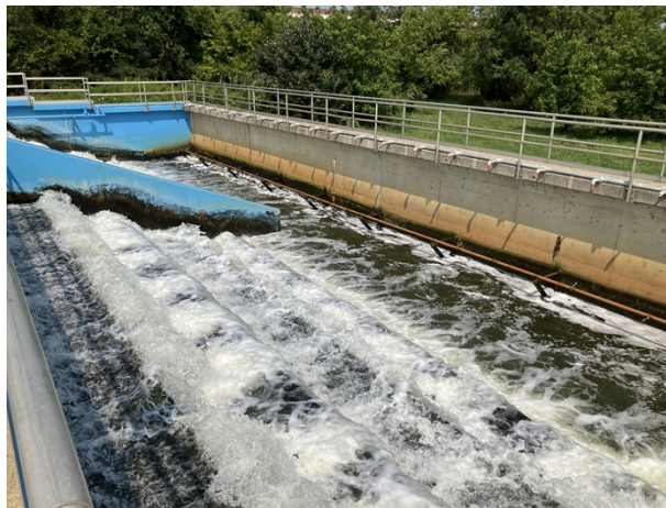
Image 03: Step Aeration system, final effluent.
