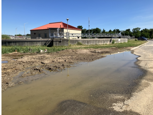
Image 06: Area of Flushing Water line break.
