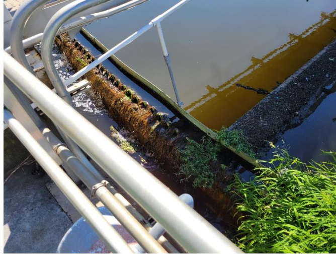
Image 4: Clarifier 8A, Scum trough clogged, excess vegetation.
