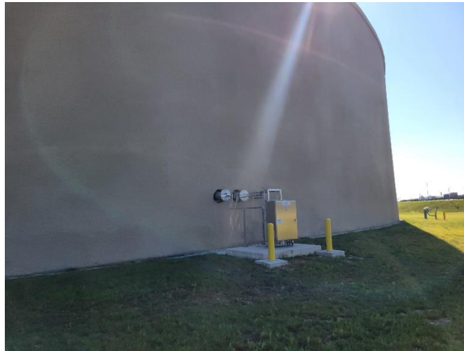
Image 6: Exterior EQ Tank 1.
