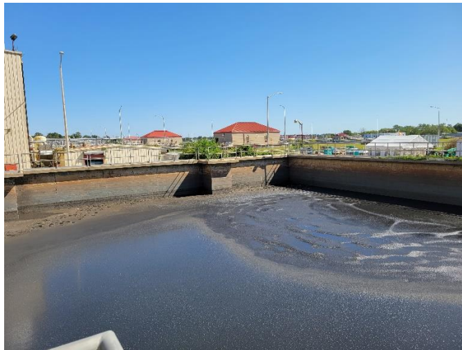
Image 2: Sludge Holding Tank, Tank 26.
