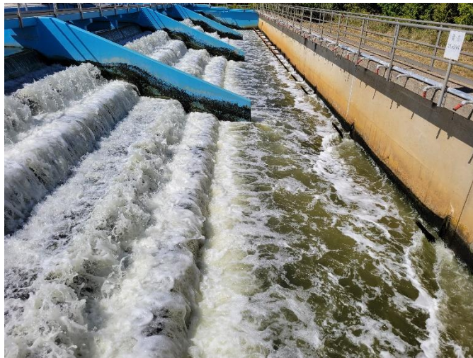
Image 5: Final effluent, Step Aeration System.
