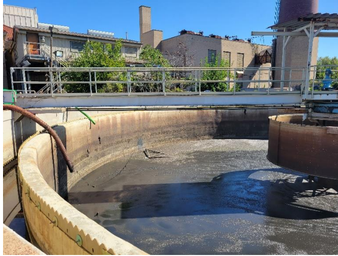
Image 1: Sludge Holding Tank, Tank 1.
