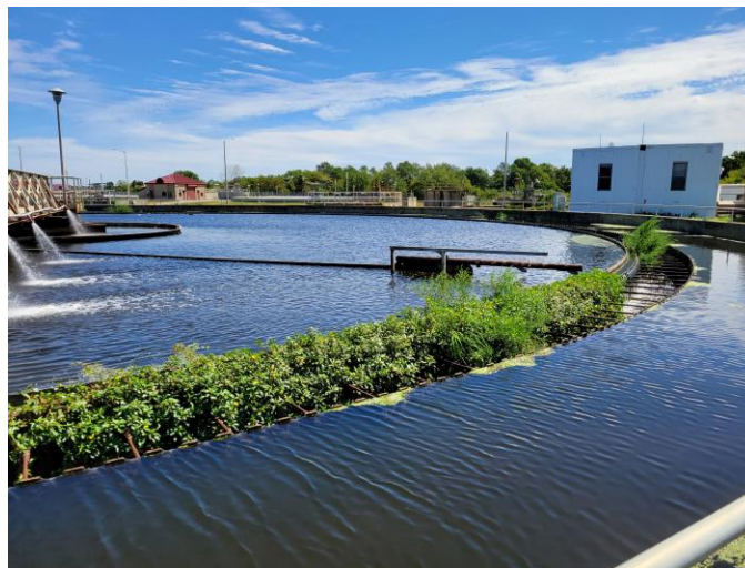
Image 3: ASP #3, Clarifier #12A, skimmer missing flap, significant vegetation.
