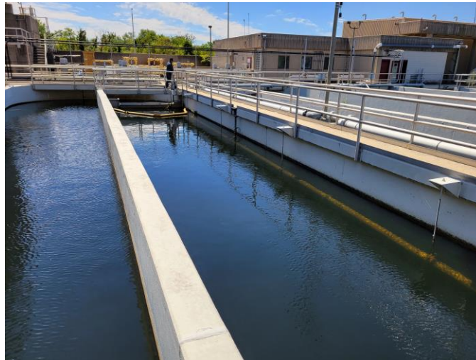
Image 4: Typical chlorine contact chamber on day of inspection.
