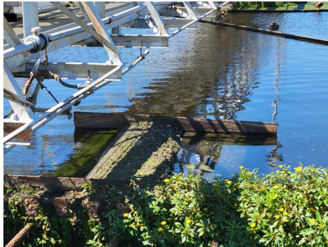
Image 2: ASP #3, Clarifier #14B, clogged scum trough, significant vegetation.
