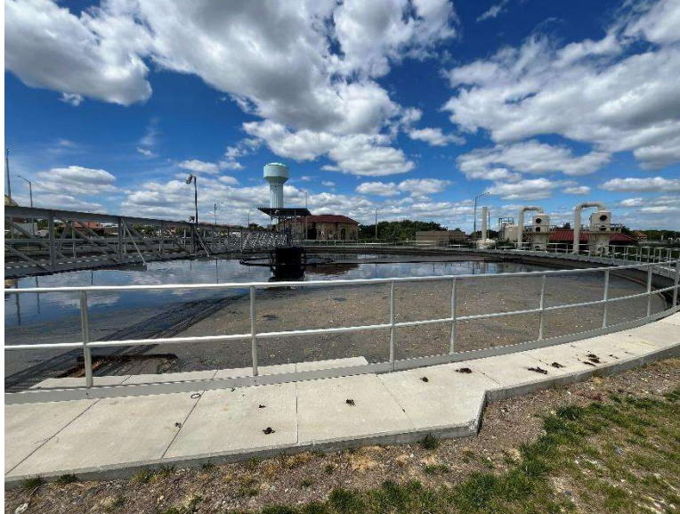
Active PST with FOG on Surface, Odor Control System in Background (Out of Service)
