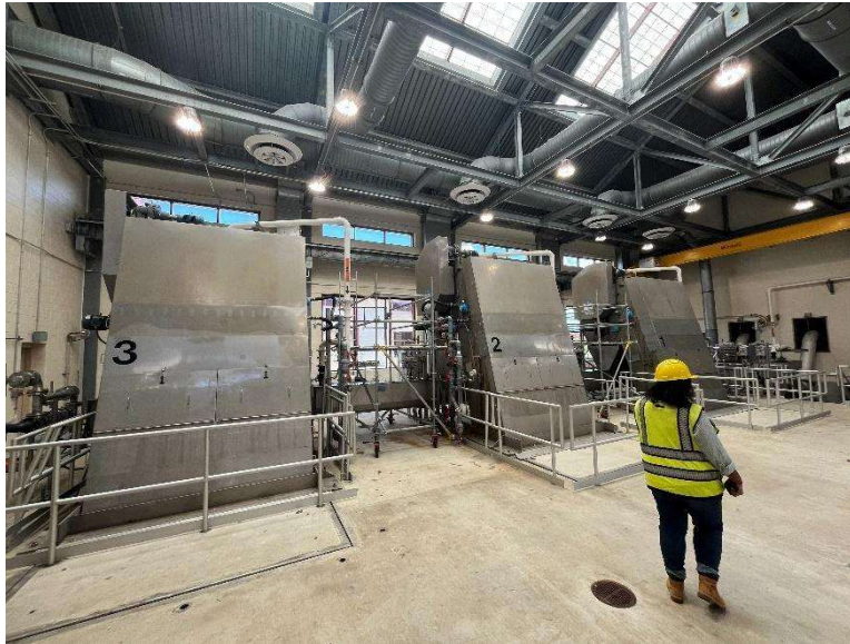
Fine Screen Facility
