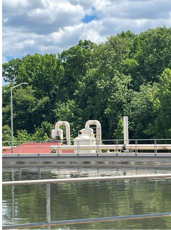
PST Odor Control System (Out of Service)
