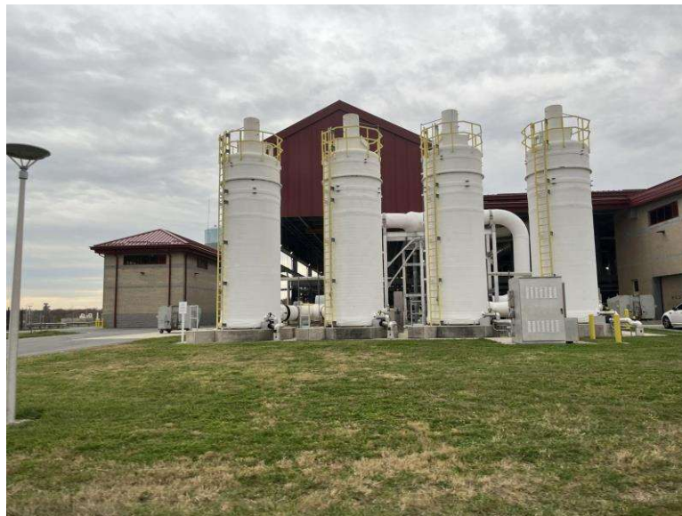
BioAir Odor Control Scrubbers
