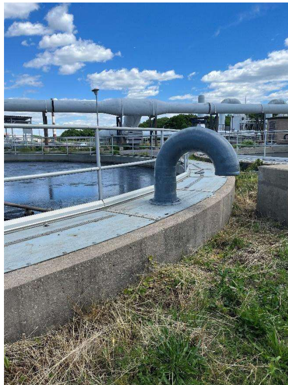
Covered Weir with Fresh Air Intake
