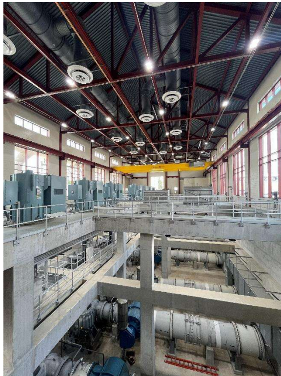
Headworks Pump Station
