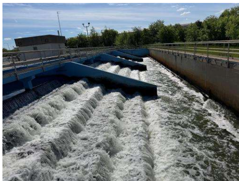
Image 06: Cascading steps with final effluent flow
