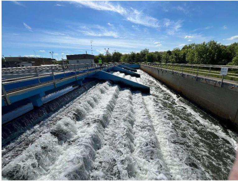
Chlorination/Dechlorination Effluent Aeration
