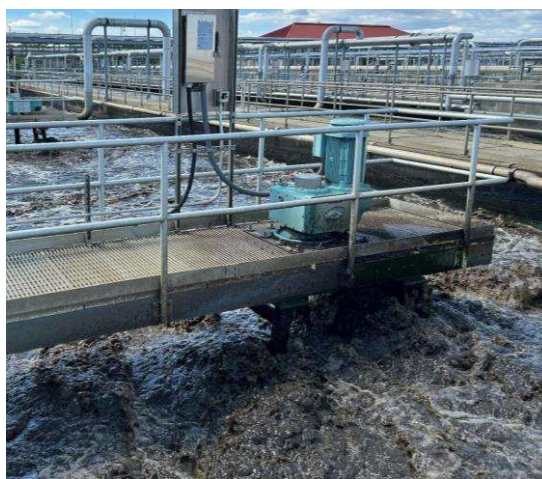
Image 05: Activated Sludge Plant 4, Pass with mixer
