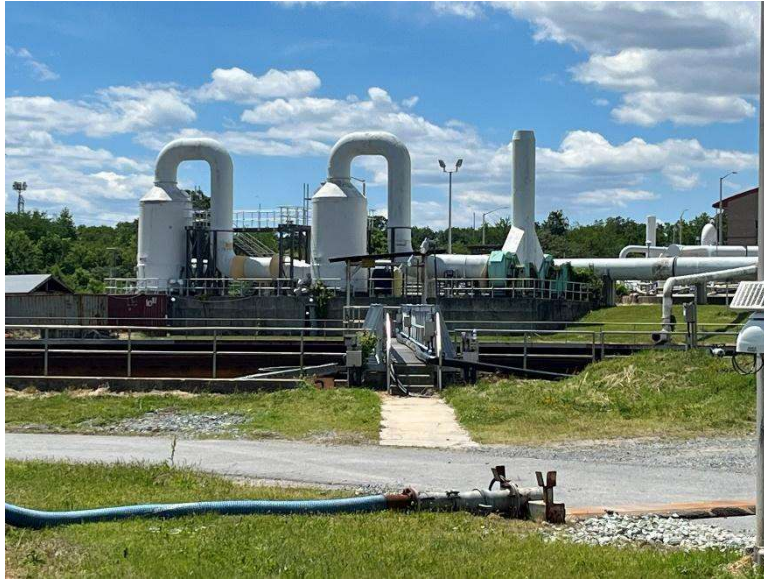
GST Odor Control System (Out of Service)
