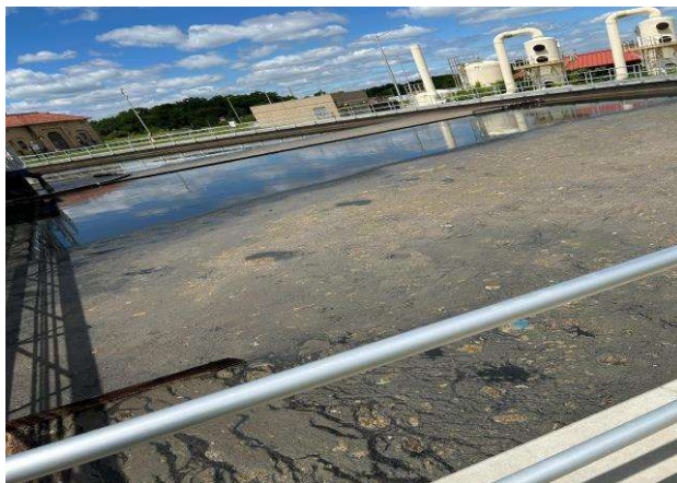
Image 03: PST 4, with a buildup of scum on top of Settling tank
