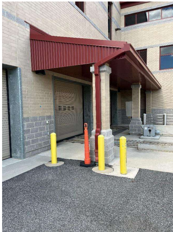
Coarse Screen Waste Loading Dock
