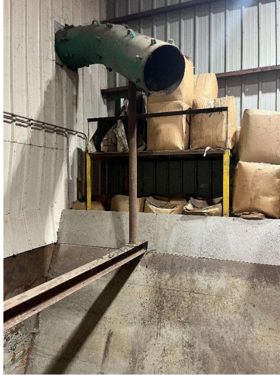
Excess Waste Dumpster Discharge
