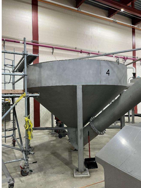
Grit Removal Cyclone
