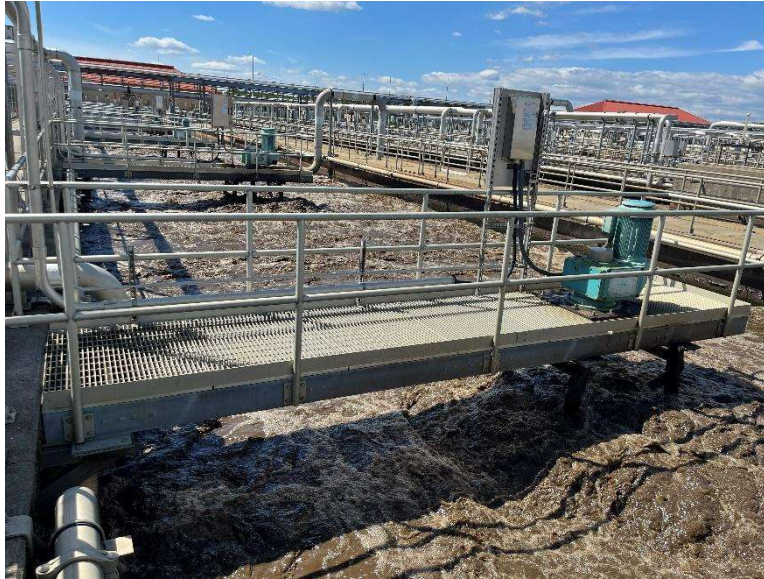
Activated Sludge Reactor
