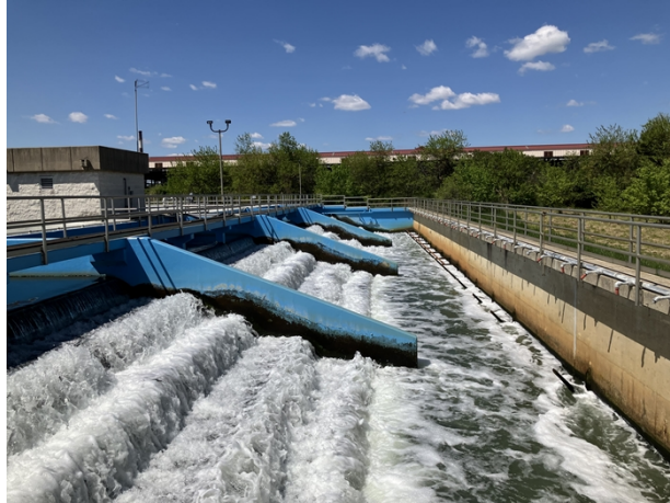
Image 02: Step Aeration system, final effluent.
