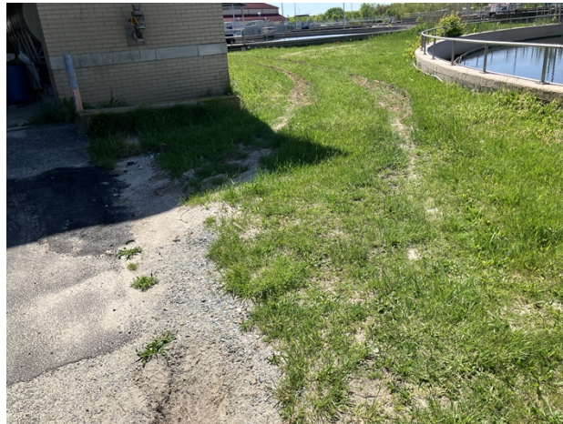
Image 04: Potable water leak area. Repaired.
