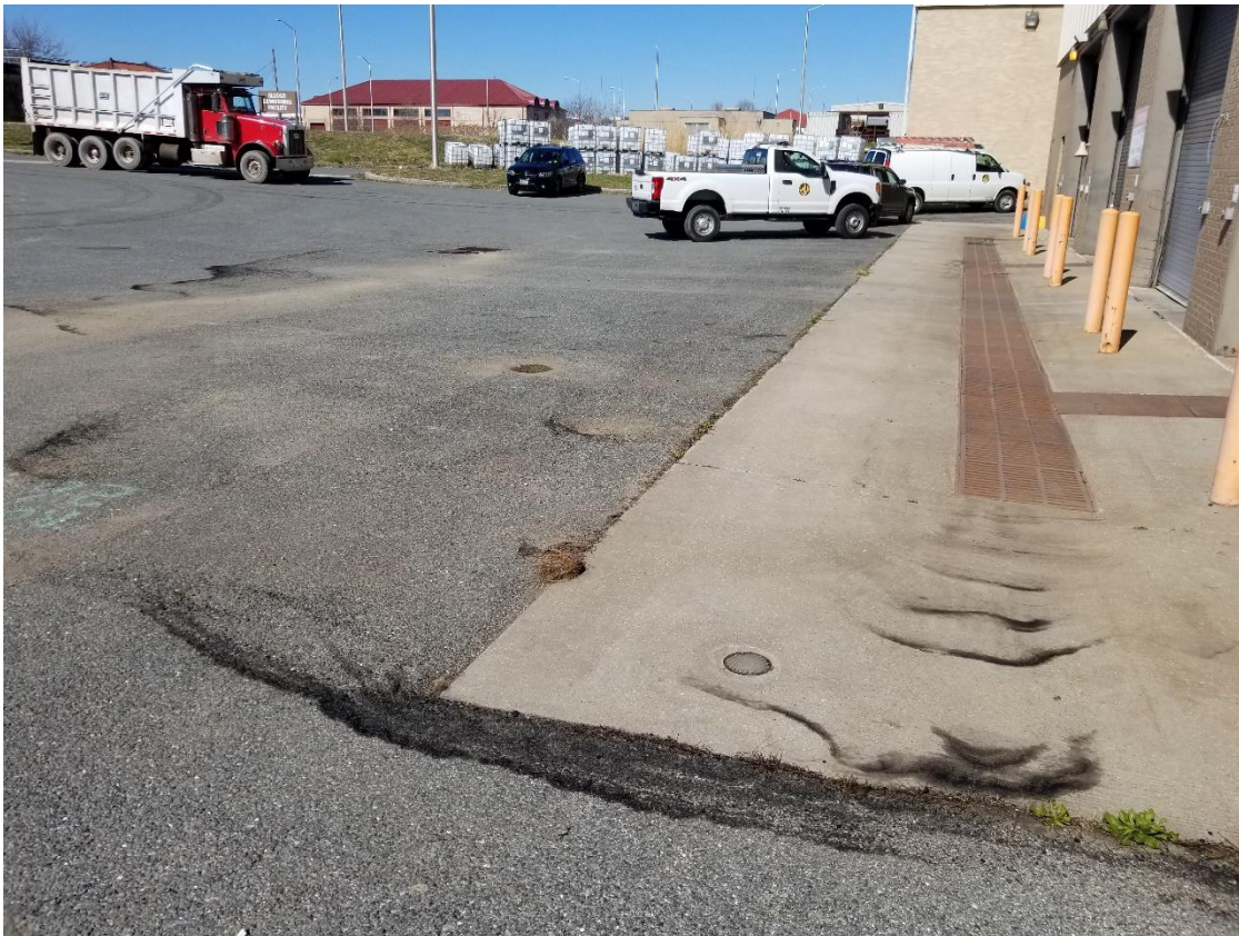
Picture 14: The area in front of the dried sludge loading building was observed to be dry.
