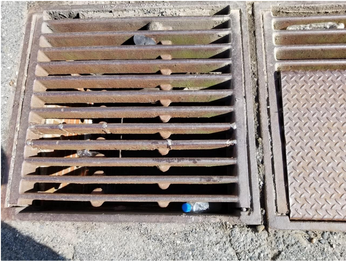
Picture 15: In front of the dried sludge loading building, no water was observed entering the storm drain inlet.
