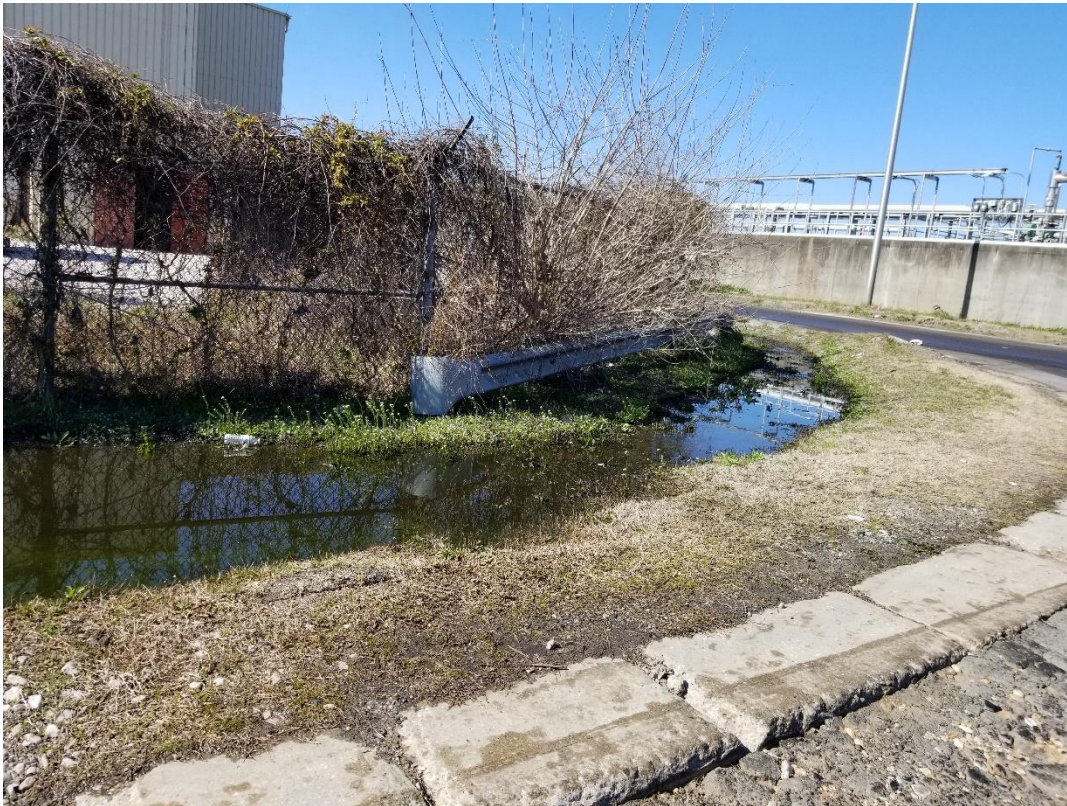
Picture 4: An oily sheen and green-ish color were observed in the flow water along the flow path from the pelletech building towards the dried sludge loading building.
