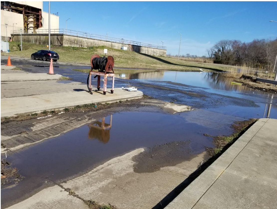
Picture 11: An area of pooled water was observed behind the dried sludge loading building past the trench drains.
