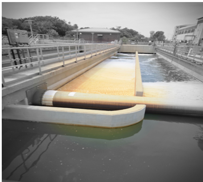
Image 05: Chlorine contact chambers (CCC #2)
