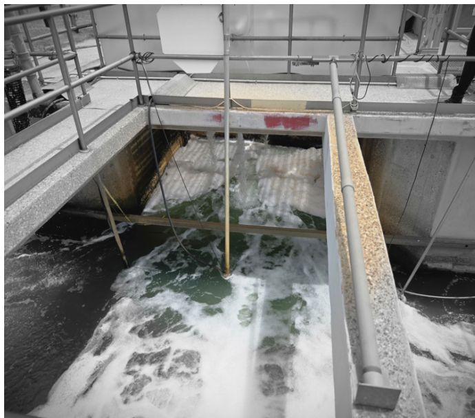
Image 06: Final effluent discharge with minimal amount of foam.
