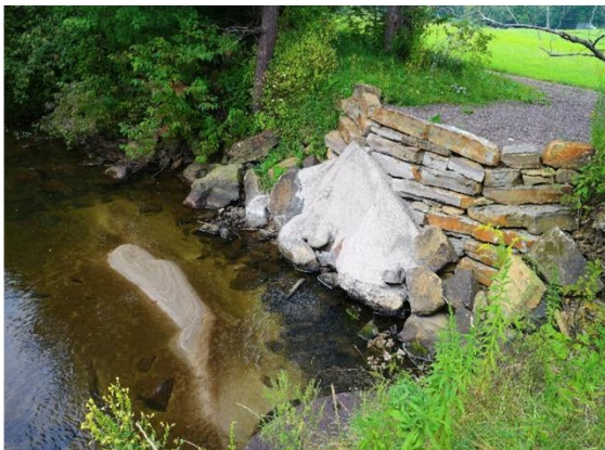
Snyder Sand Application Site Photo courtesy of MDE, Abandoned Mine Lands Division
