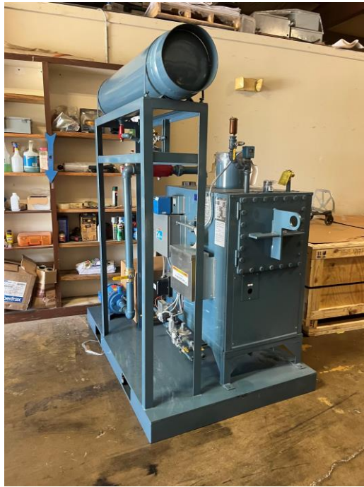
Photo C – Proposed Small Boiler to Heat Tanks (To Be Installed)
