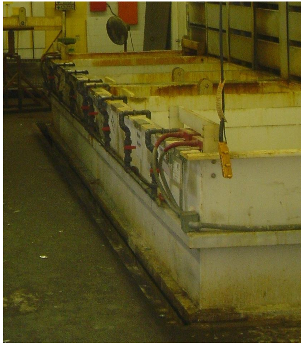
Photo A – Example of Proposed Pickling Tank (To Be Installed)
