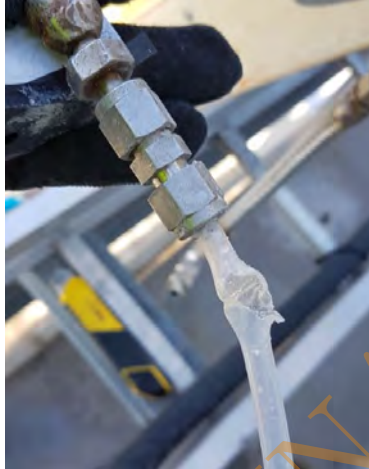
Figure 4 - Teflon tubing failure at outlet of compressor
