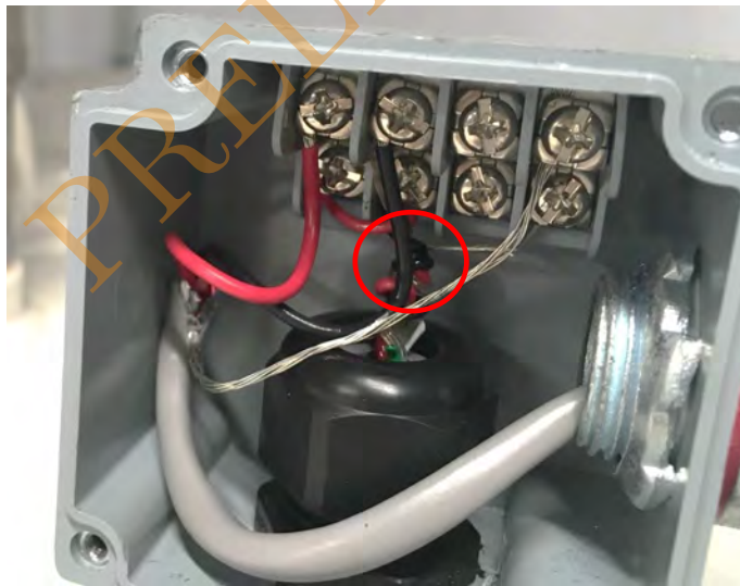
Figure 5- Potential pressure tube pinch point at level sensor junction box
