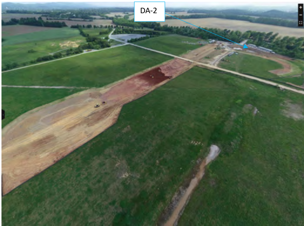
Figure 26: Start of excavation in Borrow Area for Quantum Place South – Week of 05/17/2023
