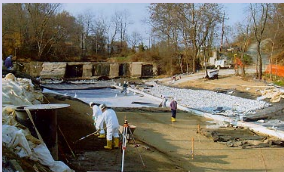
Standing in the Little Elk Creek River bed, workers prepare the subgrade for placement of the liner.
