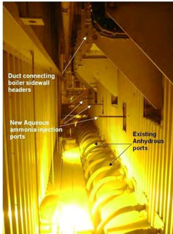
Figure 3. Tertiary Air Front Wall Duct
