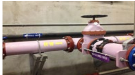
Reclaimed Water Supply Pipe at Howard County Fort Meade Reclaimed Water Pumping Station
