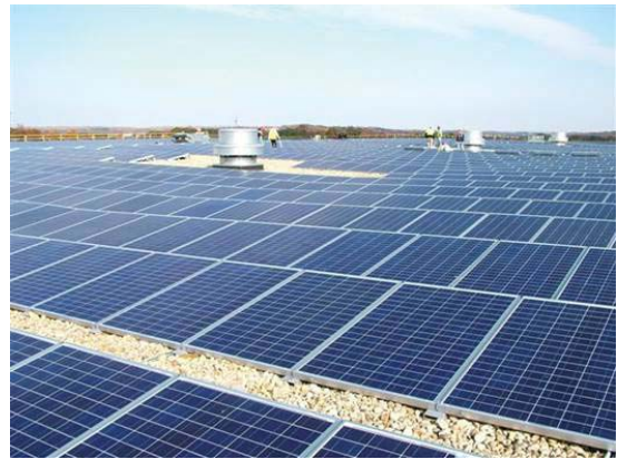
Rooftop solar array at Staples' Hanover, MD Fulfillment Center.
