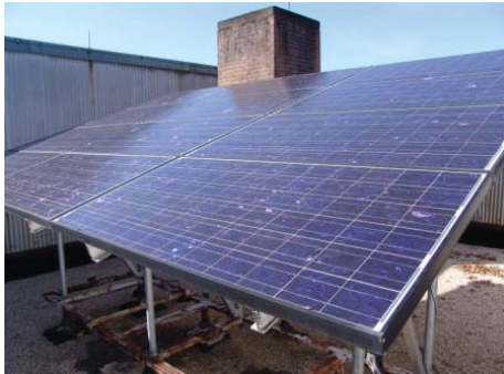
3KW photovoltaic array atop college library
